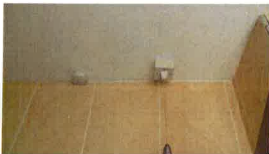
Photo 4 – Light and shower power switches
