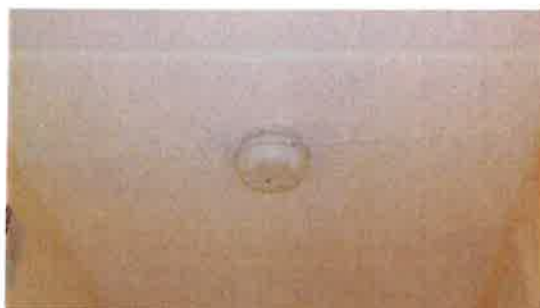
Photo 6 – Operative Hall smoke alarm
