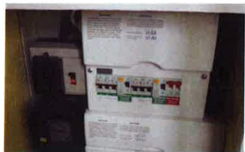
Photo 5 – Electrical switch box in hall
