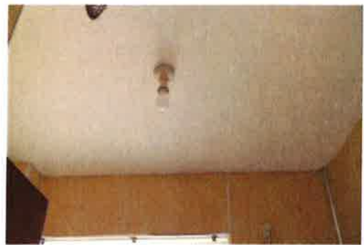
Photo 3 – B/room light fitting
