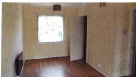
Photo 10 – New radiator in dining area
