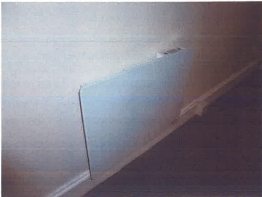
6. New electric radiant panel convector heaters in lounge and same in kitchen,
