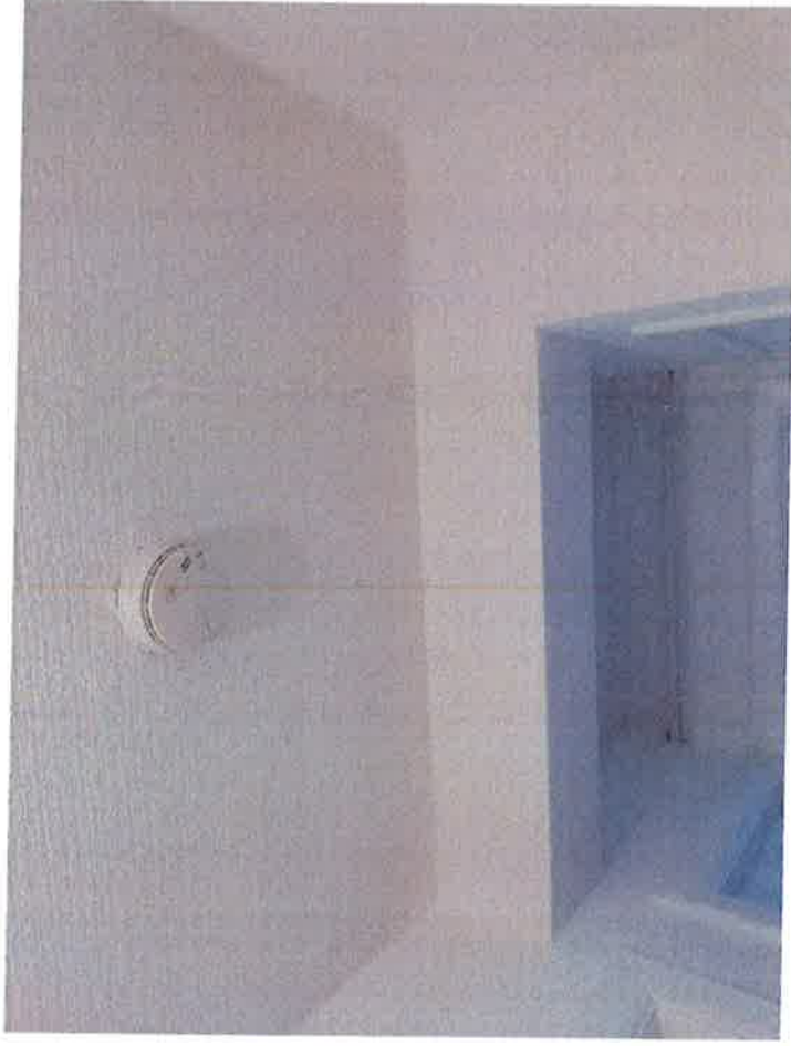
Photo 3b: as at 11/07/18 - the same device is installed, but is now connected to the new alarms in the sitting room and kitchen
