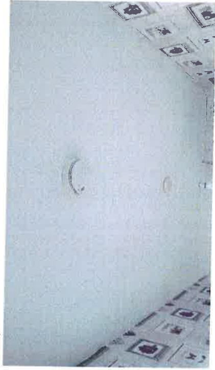
Photo 3a: smoke alarm in hall as at 12/08/16
