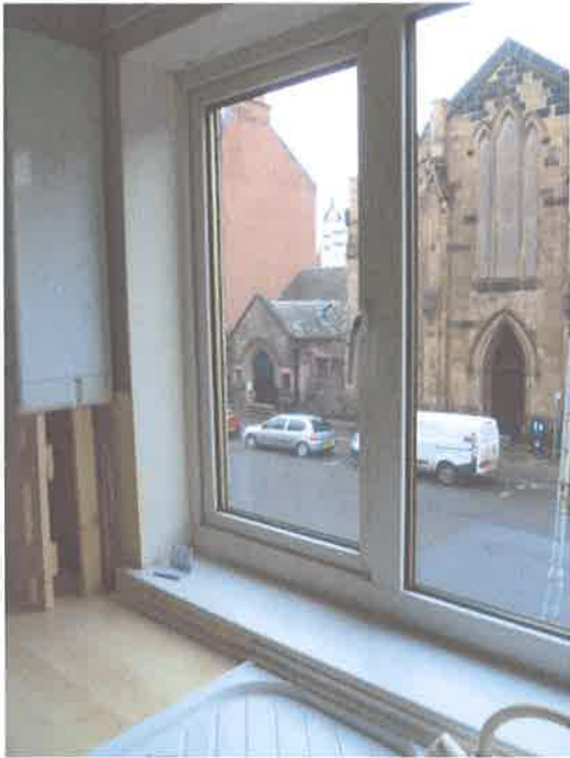
Kitchen window February 2017
