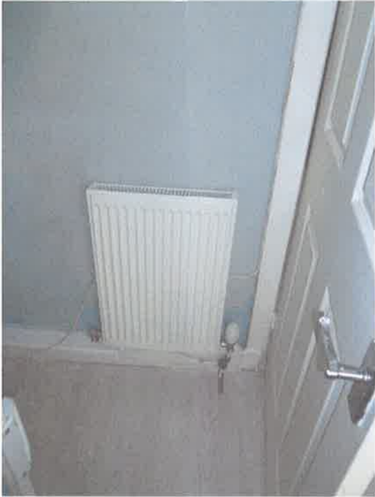
Kitchen radiator February 2017
