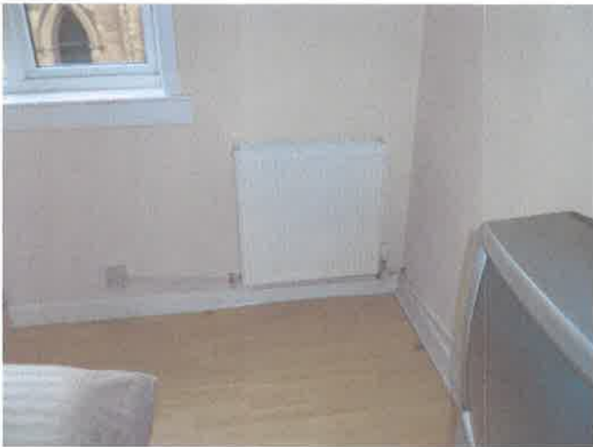
Bedroom radiator February 2017
