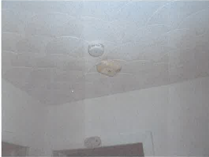
Smoke alarm to hall February 2017
