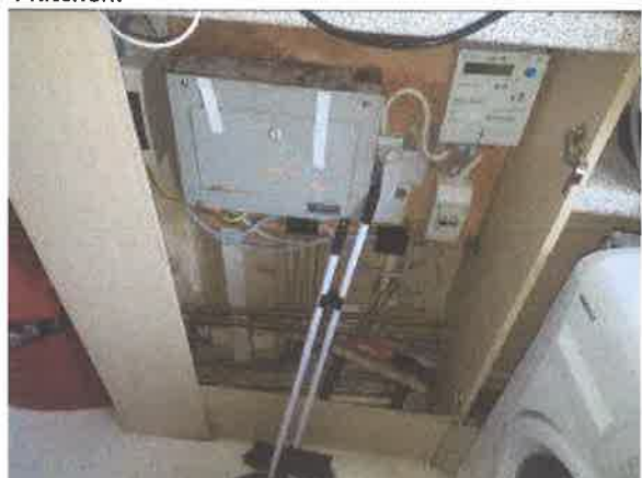
6 Electrical Consumer Unit.
