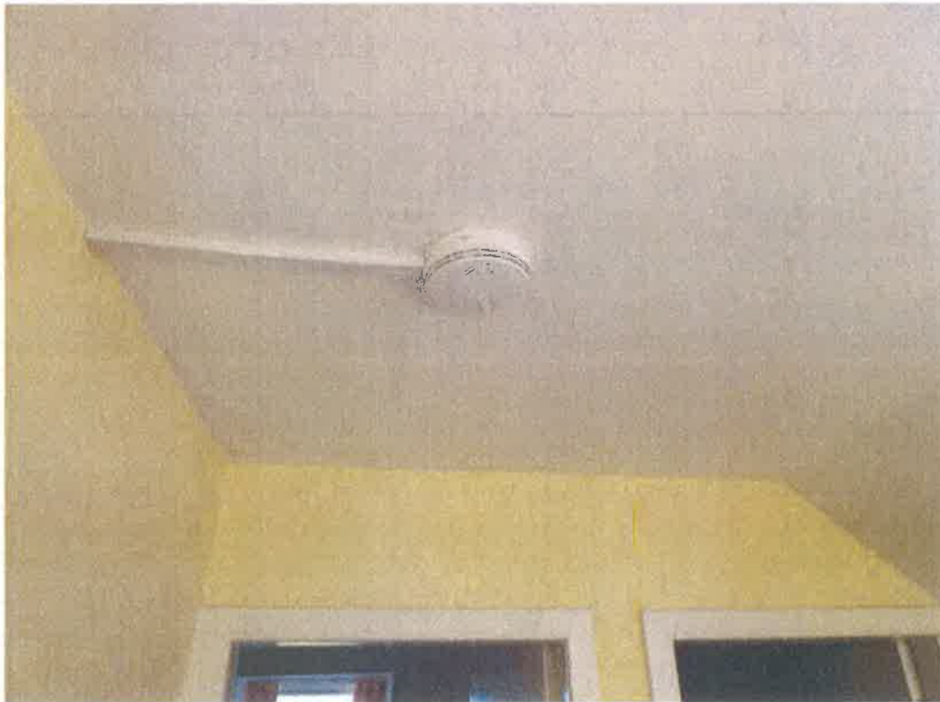
Internal view of flat roof over landing where leak occurred previously. Dry plaster re-decorated before recent heavy rain
