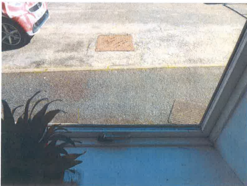
Front kitchen window – lower section – catch
