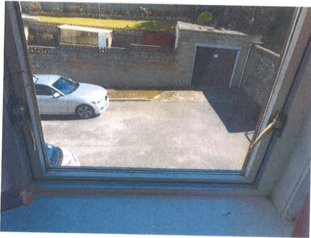
Front 1 st floor bedroom window - catches
