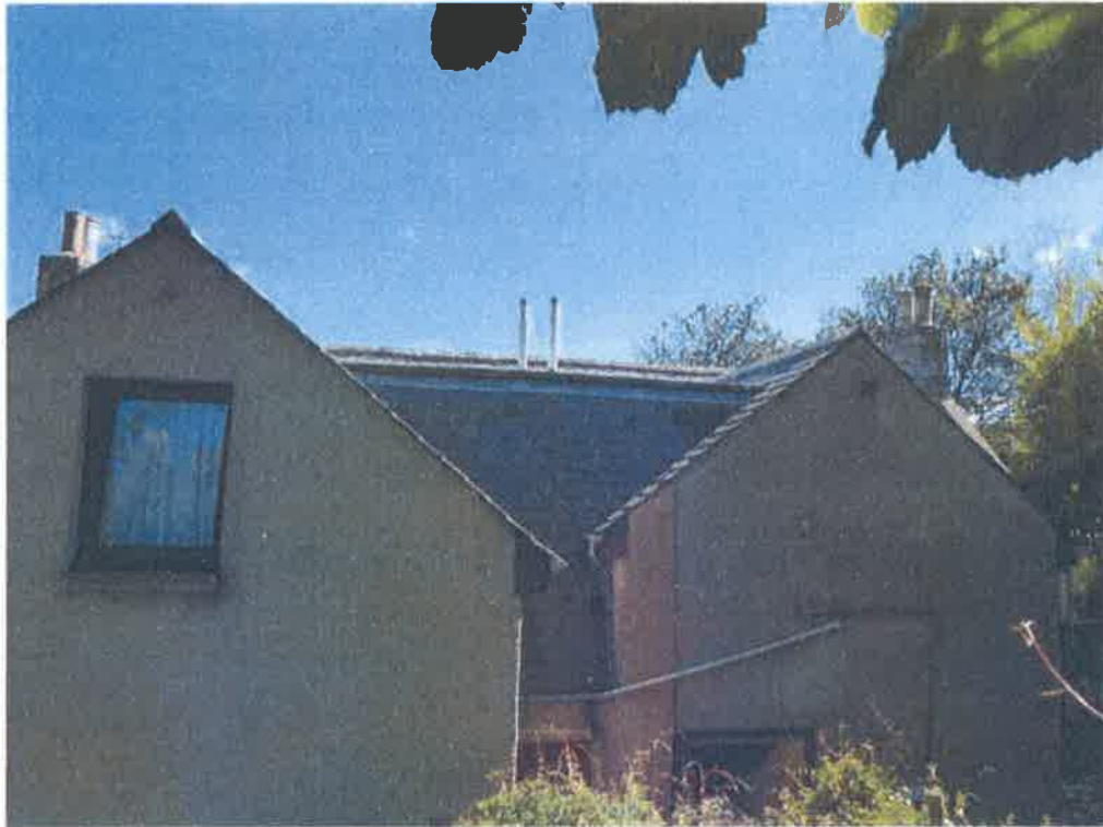
External view of flat roof. Not possible to find a higher point to see actual flat roof covering.
