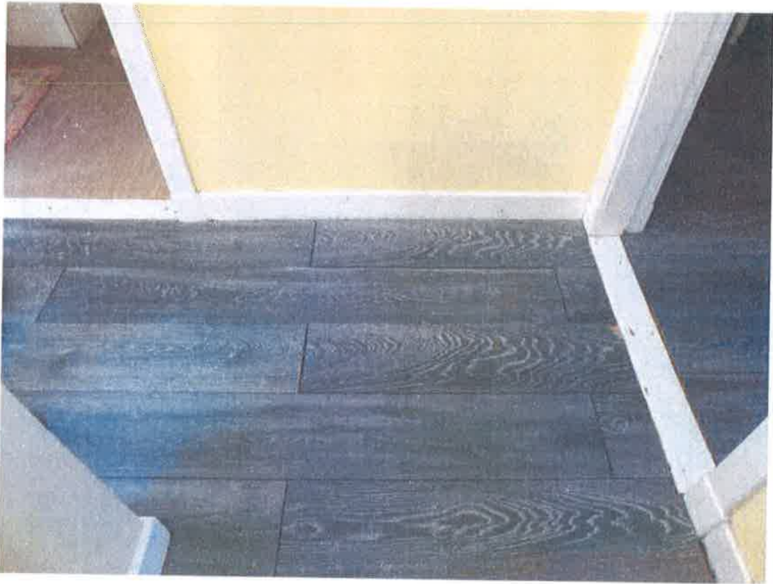
Laminate floor to landing which is loose. Sections easily moved
