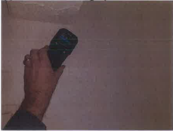
1 High moisture readings above entrance door.
