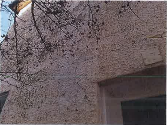
10 Gable elevation – cracking remaining to render.
