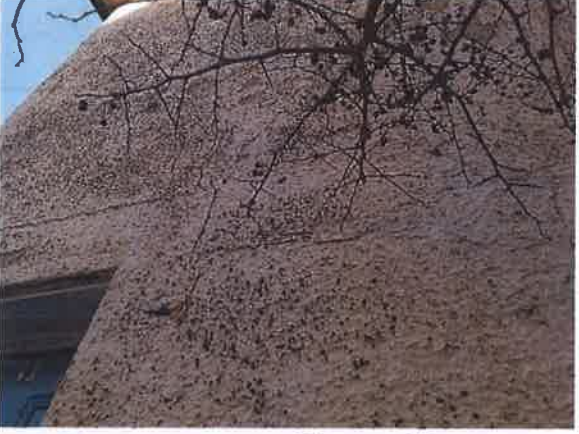
12 Gable elevation – cracking remaining to render.
