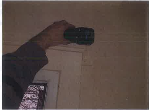
2 High moisture readings above entrance door.
