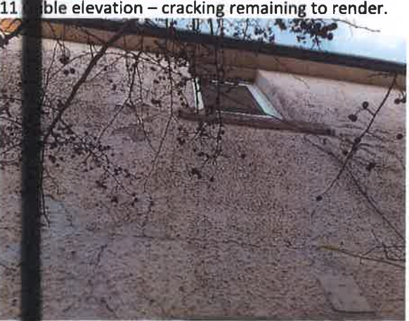
13 Gable elevation – cracking remaining to render.
