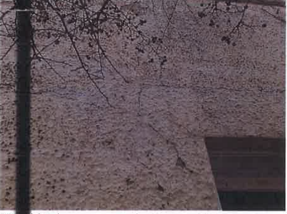
11 Gable elevation – cracking remaining to render.
