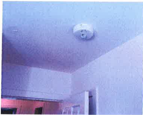
Heat alarm kitchen 29-10-18
