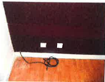
03 - Living room - power socket and TV socket
