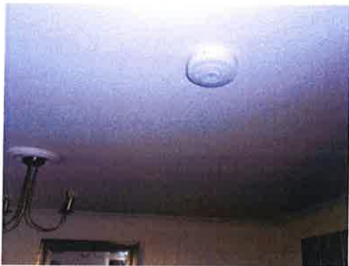
Smoke alarm living room 29-10-18
