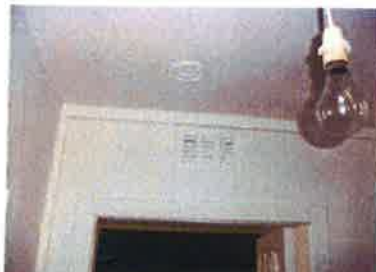
02 - Hall - bracket for battery-operated smoke detector
