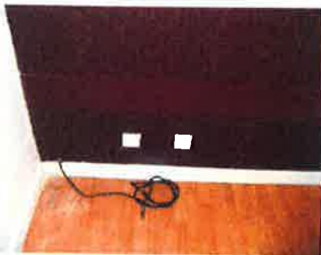
03 - Living room - power socket and TV socket
