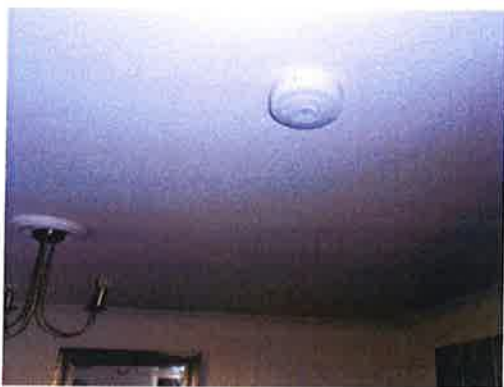
Smoke alarm living room 29-10-18
