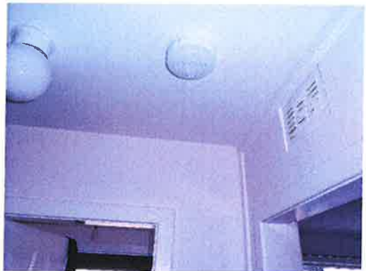
Smoke alarm hallway 29-10-18
