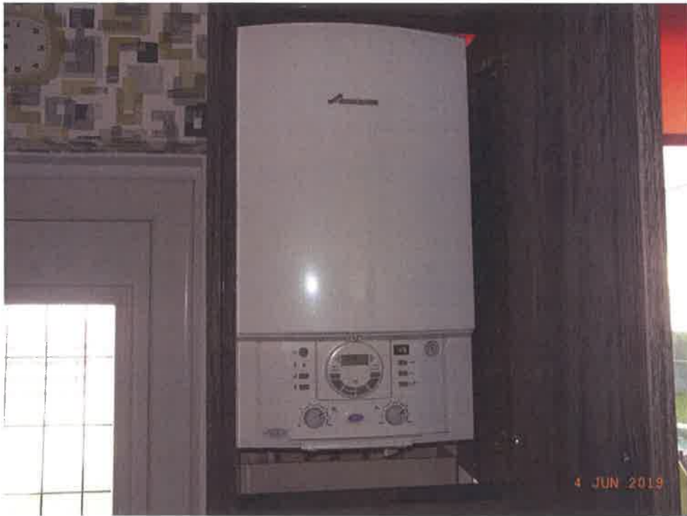
Replacement central heating boiler
