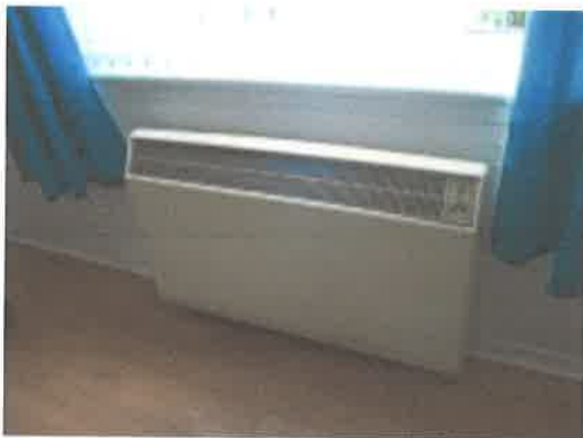
LIVING ROOM RADIATOR
