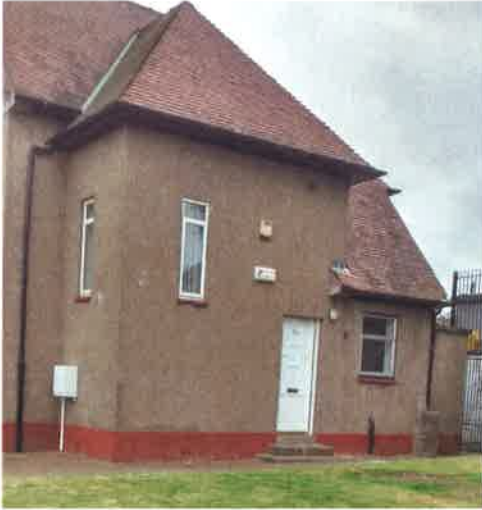
Photo 1: Front elevation – note damage to roof to right of door – but no internal evidence of water penetration
