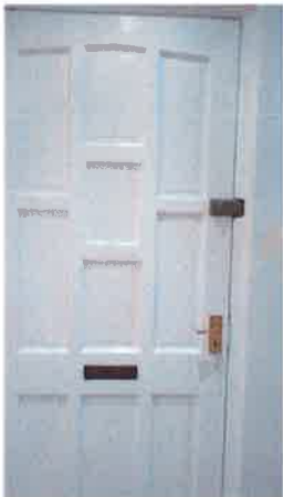
Photo 3: front door is wind and watertight with satisfactory seals
