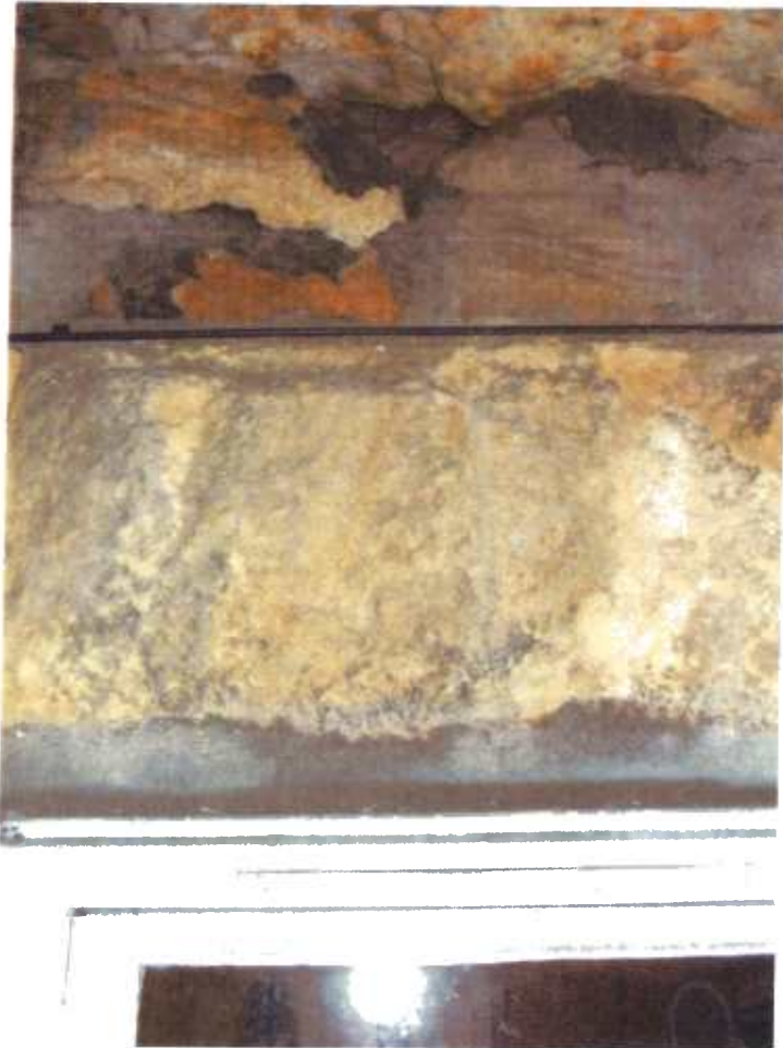
Gap in External Stonework above Window
