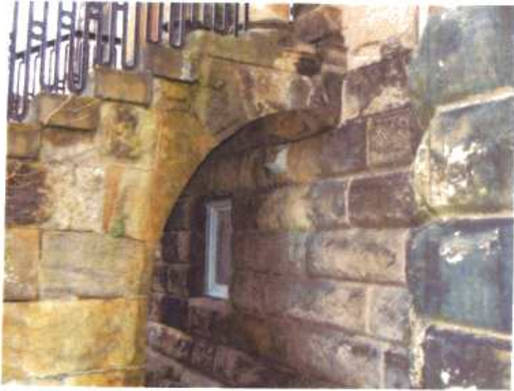
Bedroom Window – Below External Stair to Upper Flat
