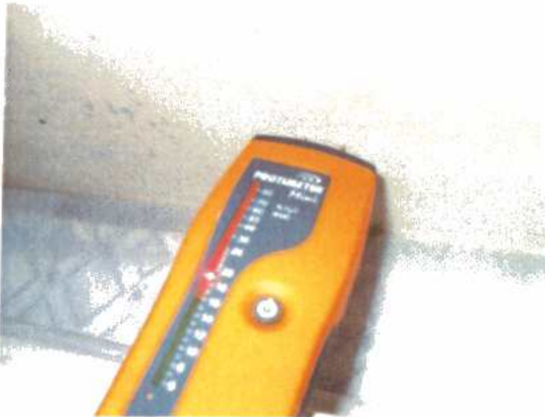
Damp Meter – Bedroom Rear Wall
