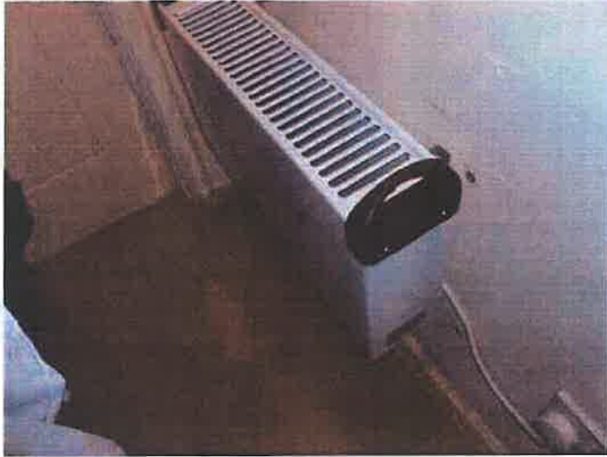
5. Panel heater – hall.
