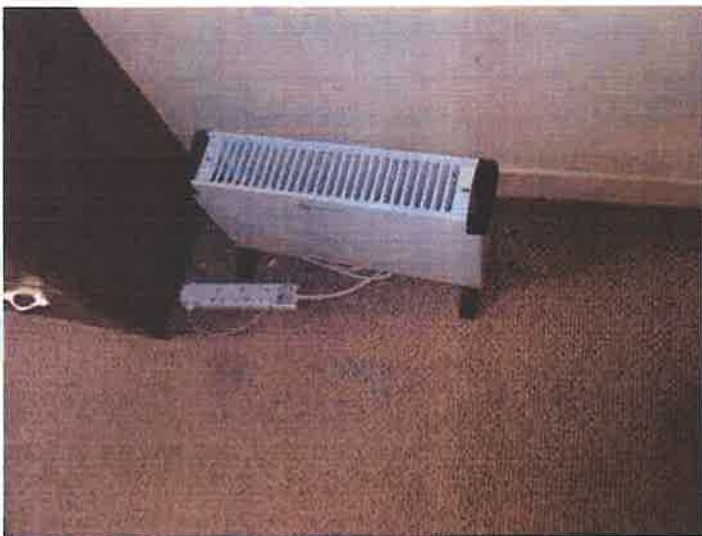
6. Panel heater – bedroom 1.
