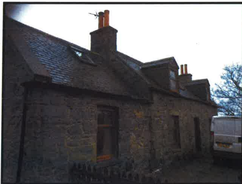
Figure 3 Front elevation left hand side - all guttering replaced, replacement windows, replacement chimney cans.
