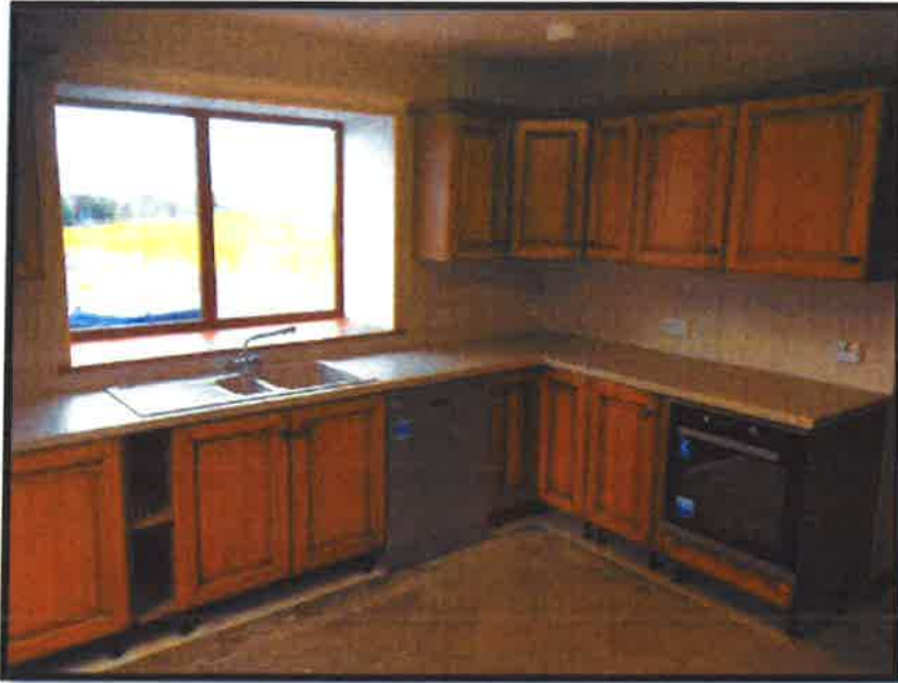
Figure 8 Kitchen - New cabinets, worktops and electric oven installed. New window and linings, typical throughout house.
