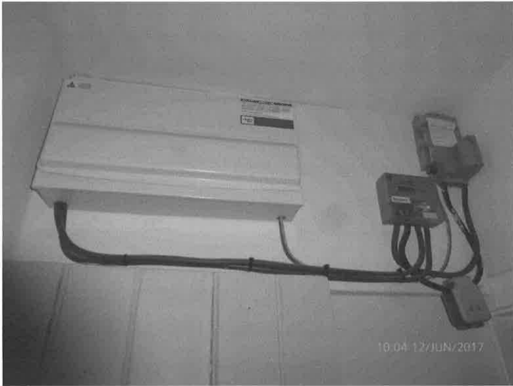
New electrical installation
