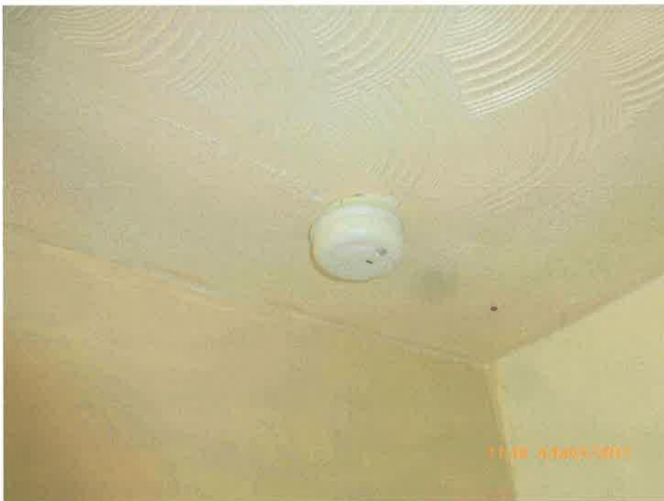
Smoke detector in the living-room
