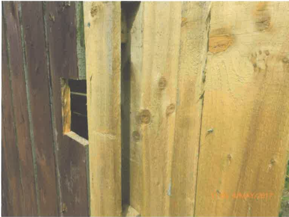
Protruding screw on gate
