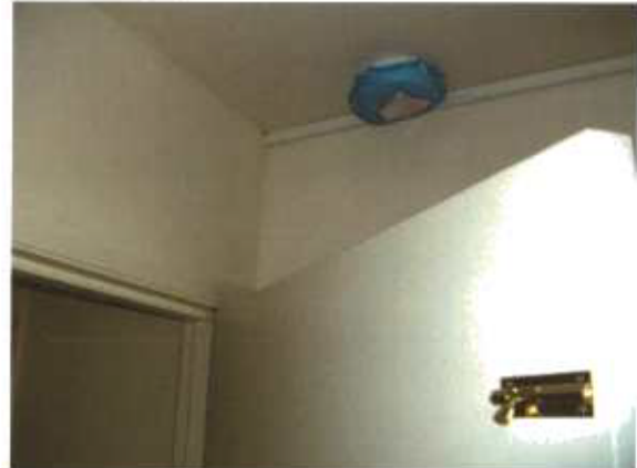
04 - Heat detector - kitchen
