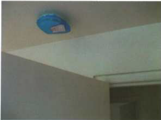
03 - Smoke detector - living room
