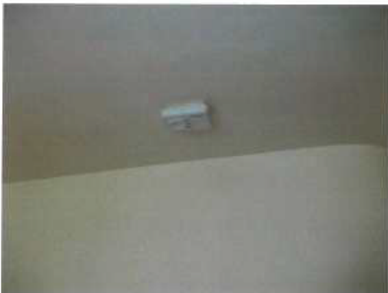
05 - Carbon monoxide alarm - kitchen
