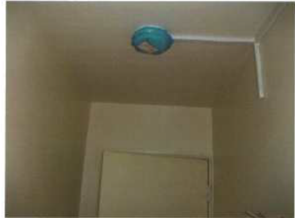
02 - Smoke detector - hall
