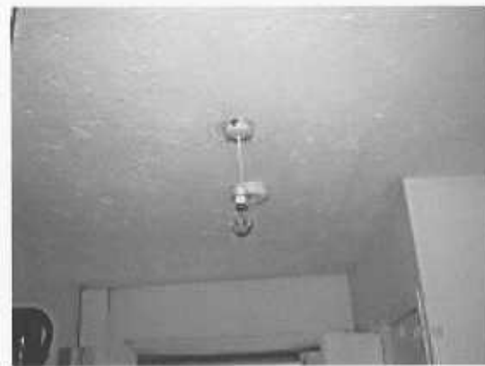
Smoke detector/light fitting
