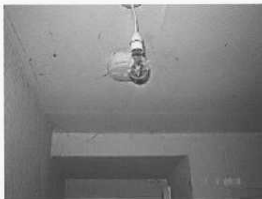
Smoke detector/light fitting
