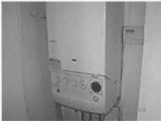
Central heating boiler
