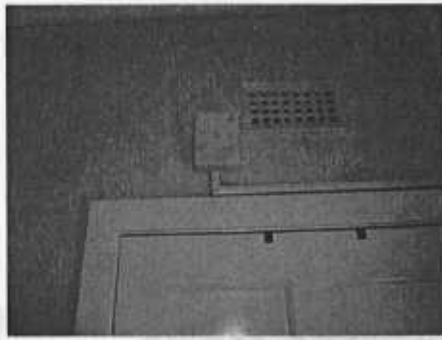
6. Carbon monoxide detector, hall
