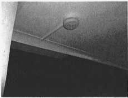
5. Hard-wired smoke detector, living room
