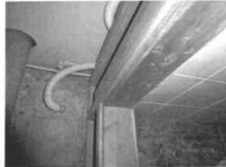
Non connected pipe
