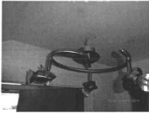
Loose light fitting
