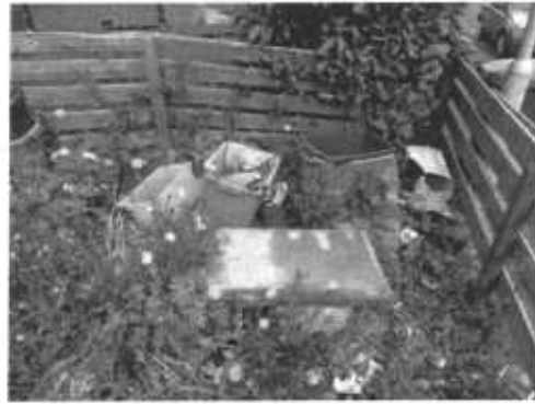
Loose manhole covers
