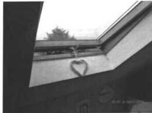
Mould below skylight window
