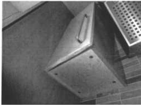
Delaminating wall unit
