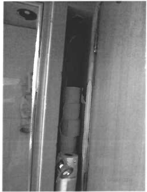
Dangerous light fitting
