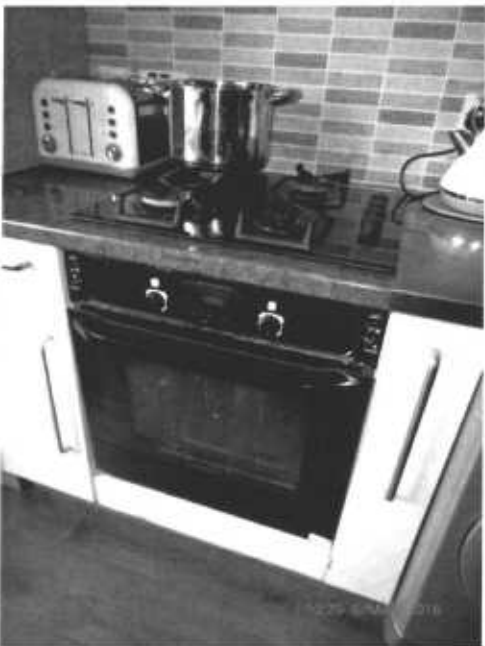
Missing front panel on cooker
