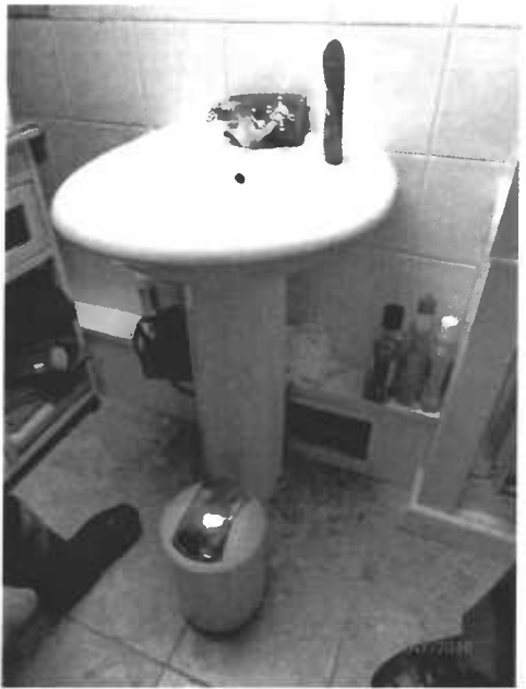
Loose wash hand basin
