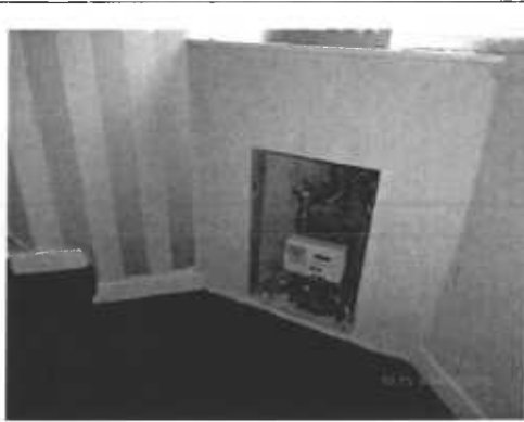
No cover on gas meter box
