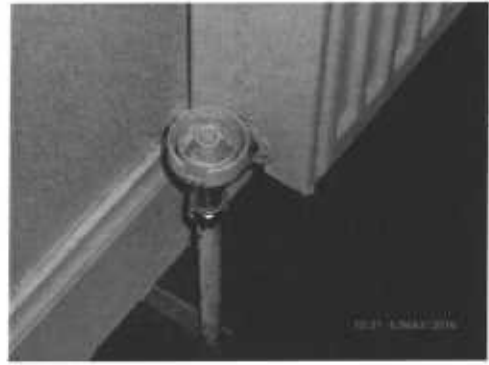
Missing thermostatic radiator valve
