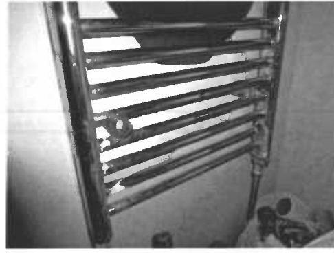
Rusting radiator towel rail
