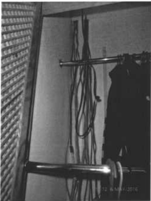
Loose/dangerous wiring in wardrobe
