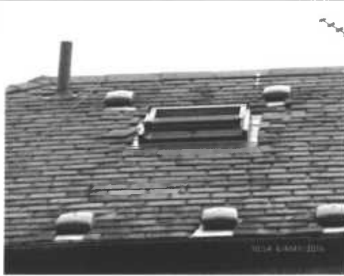
Detail showing loose/missing slates
