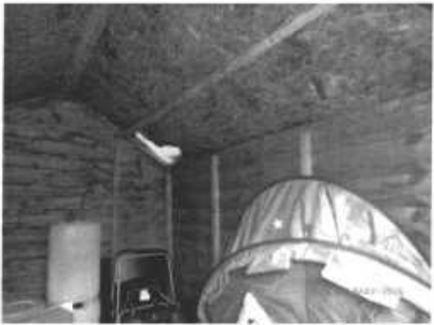
Hole in roof of shed
