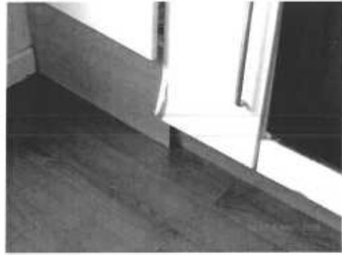
Delaminating base unit
