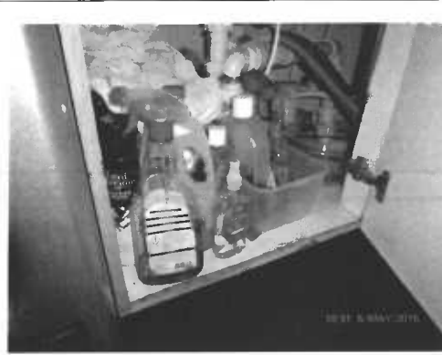
Leak below sink
