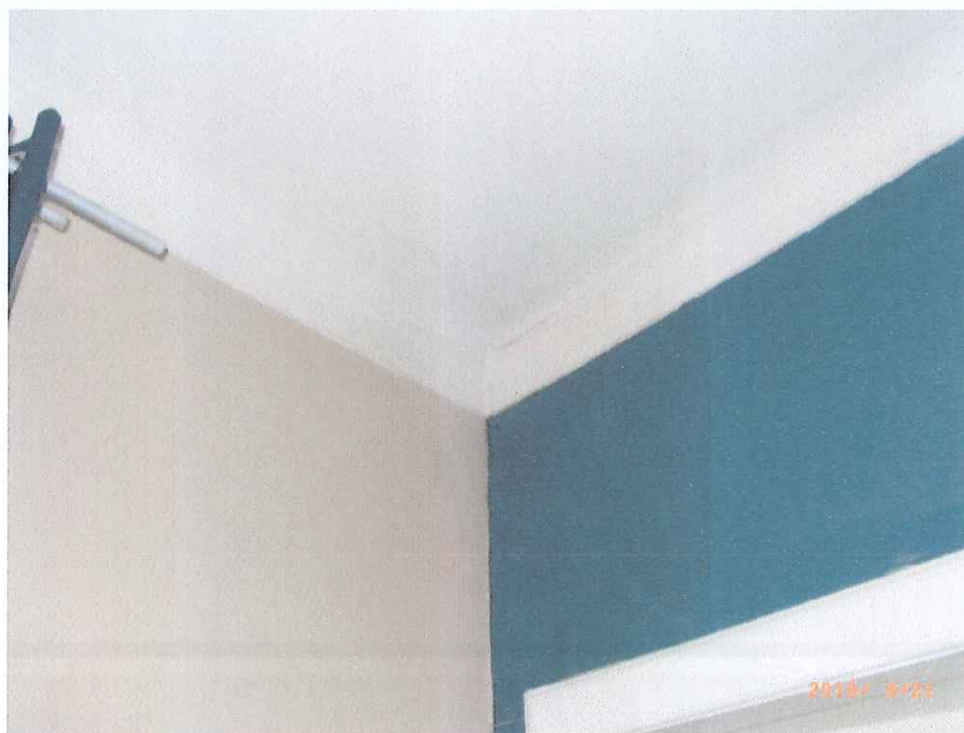
Condensation affecting upper wall/ceiling of Bedroom
