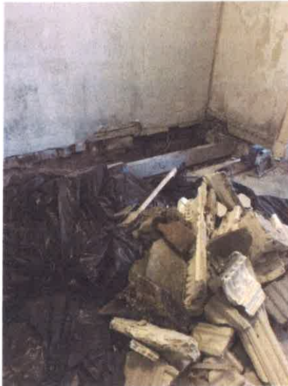
Photographs 2 and 3: Living room – wall and floor
