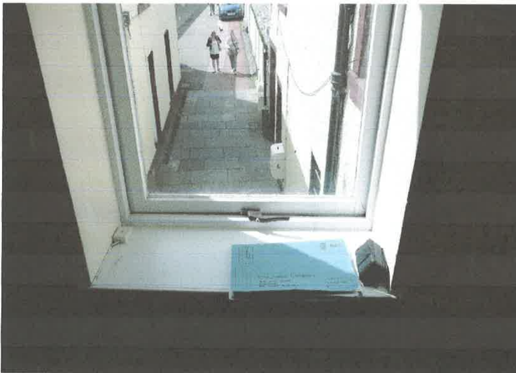
Bedroom window in closed position – catch failed and wide gap to left hand side
