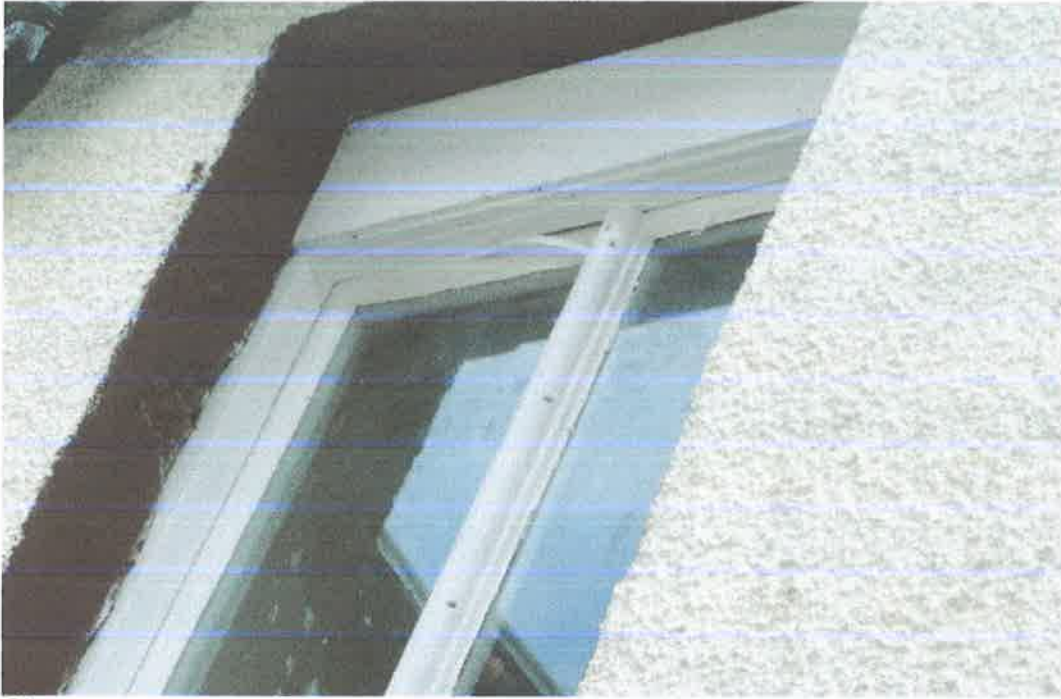
Close up of kitchen window with top draught proof strip out of position and adrift.
