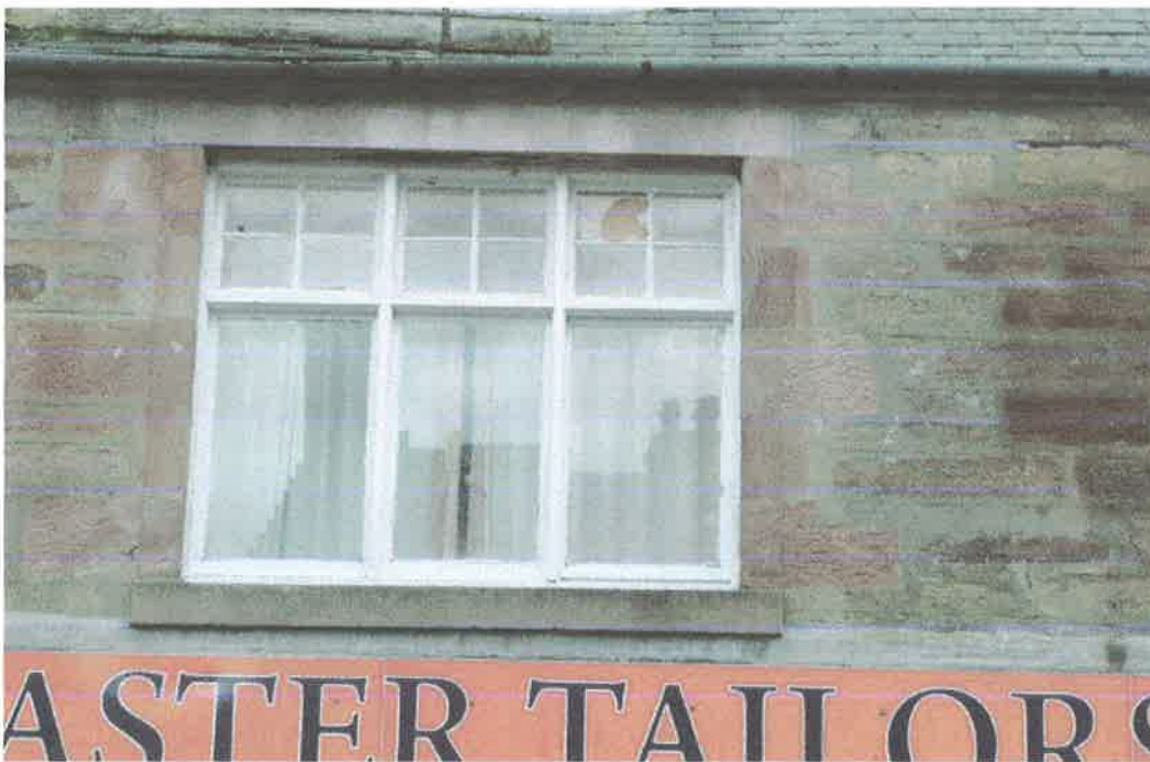
Close up of damaged window. Cracked central pane and broken top right pane.
