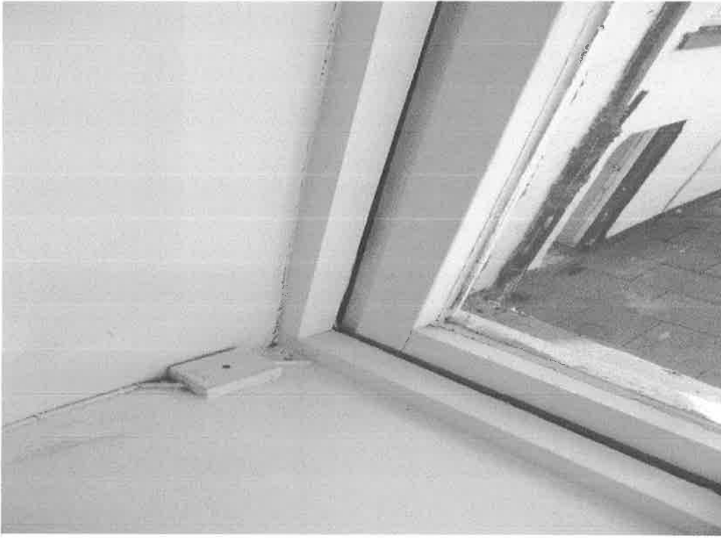
Bedroom window left side showing gap at base level
