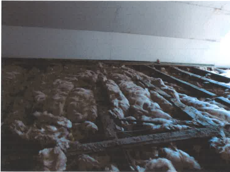
Insulated loft space. All floorboards have been lifted and quilt insulation laid between joists
