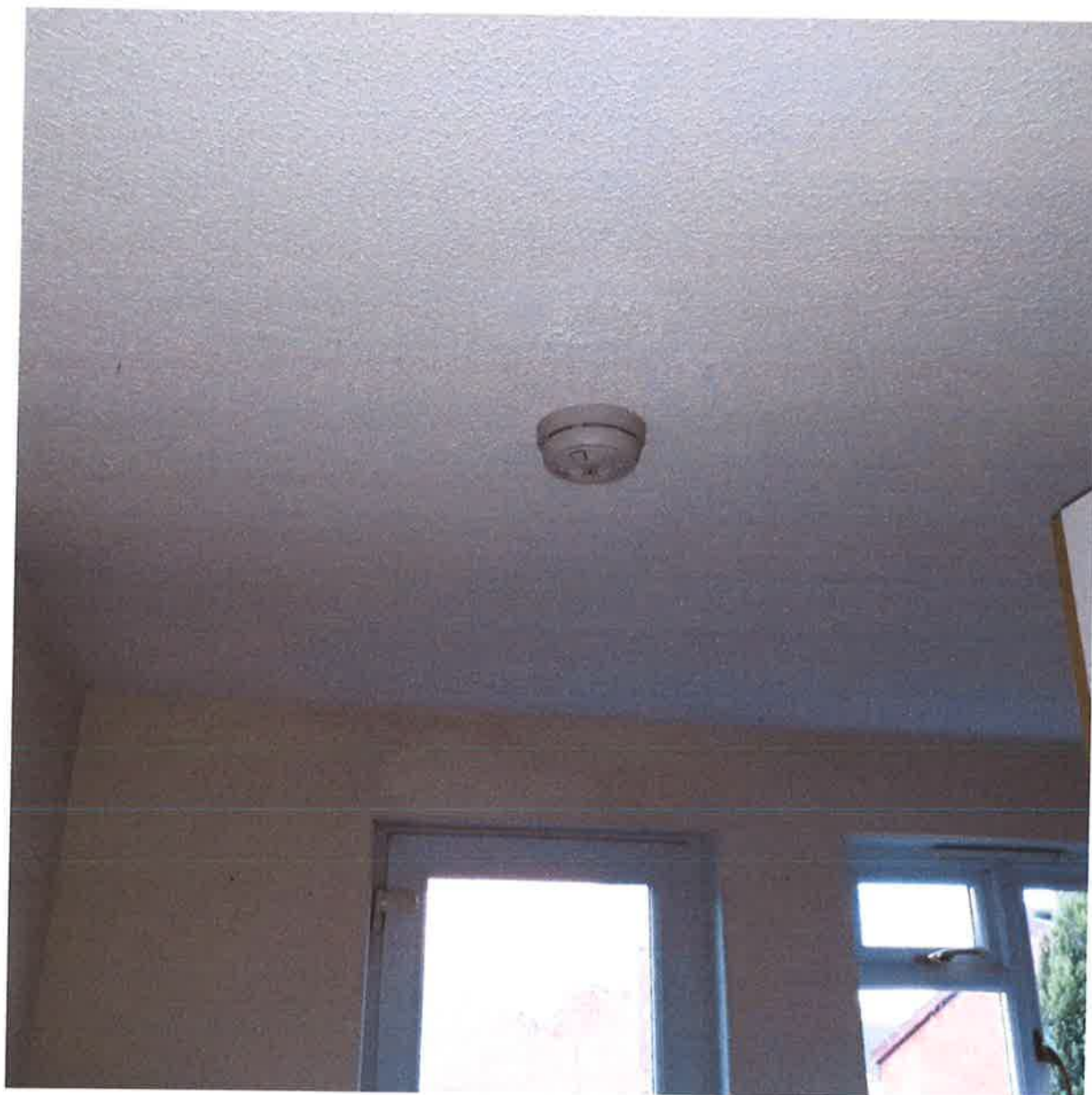
5 View of newly fitted hard wired heat detector in the kitchen.
