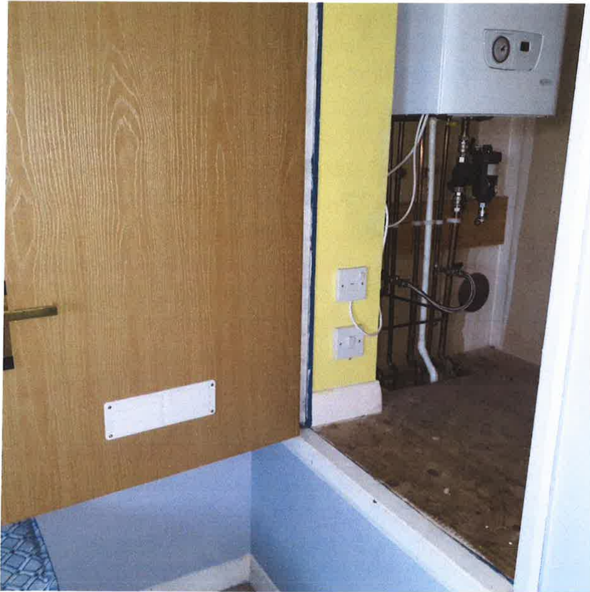
4 View of the boiler cupboard. Ventilator fitted awaiting fitting of a CO2 detector in the adjoining bedroom
