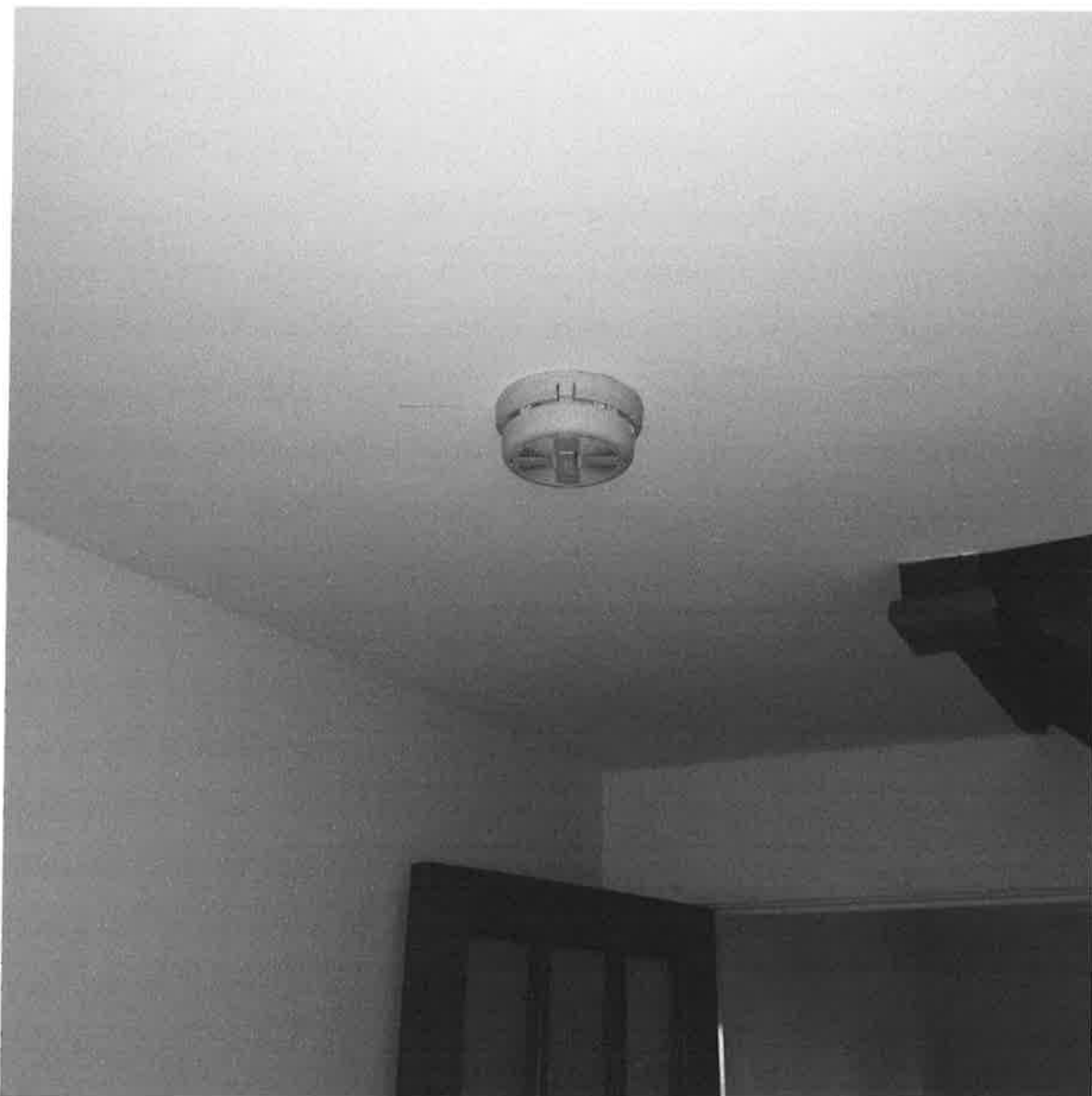
2 View of the repaired lounge ceiling and newly fitted hard wired smoke detector
