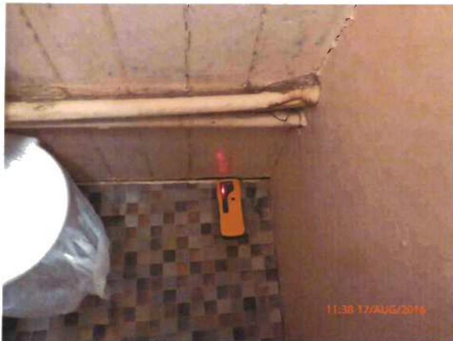
Dampness in the bathroom
