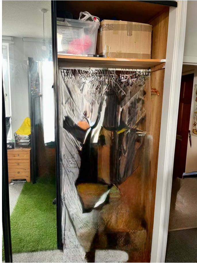
Missing wardrobe doors
