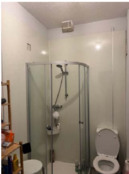
Shower-room showing inaccessible air vent
