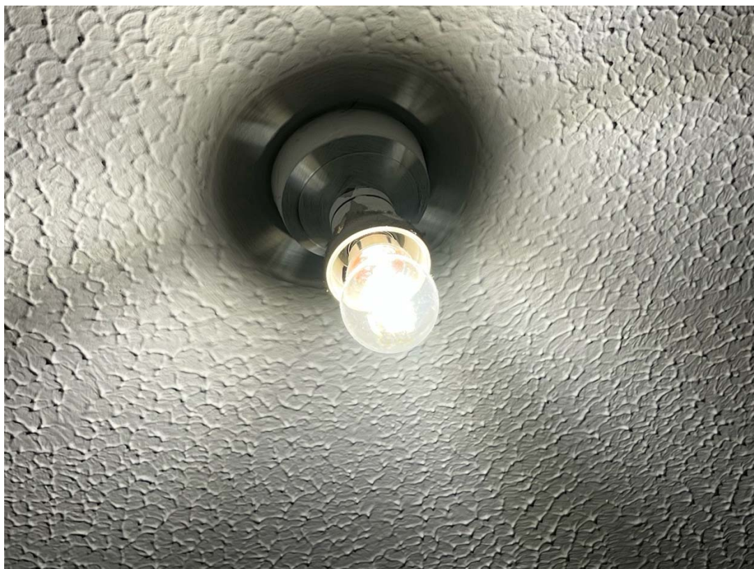
Exposed light bulb in the shower-room
