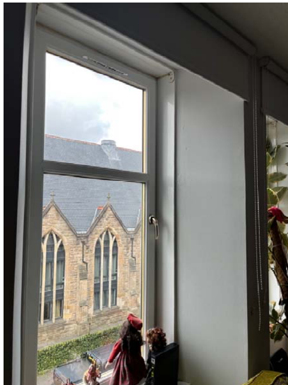
Broken blind cord
