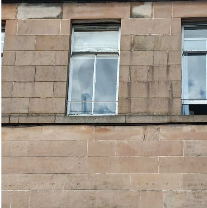
2 Kitchen window, Flat 5 (LHS pane cracked)
