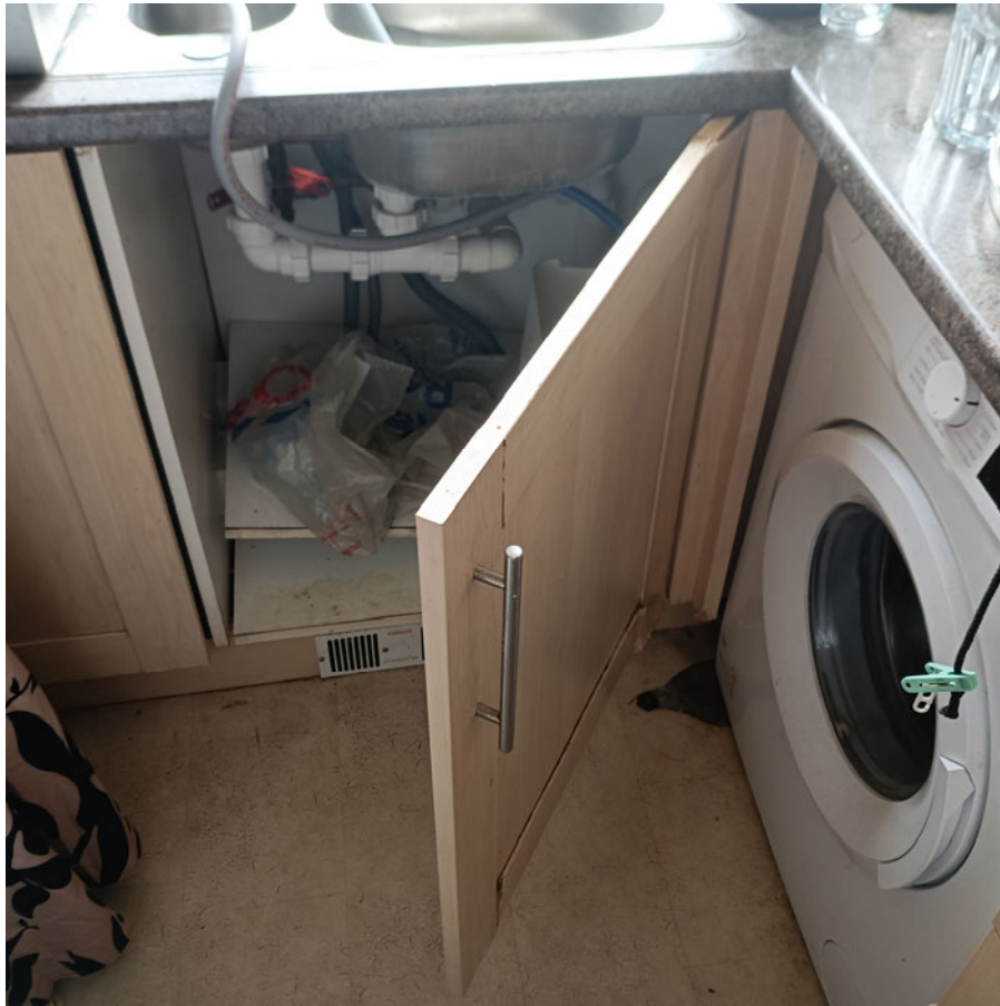
6 Damaged under sink store cupboard door and shelving
