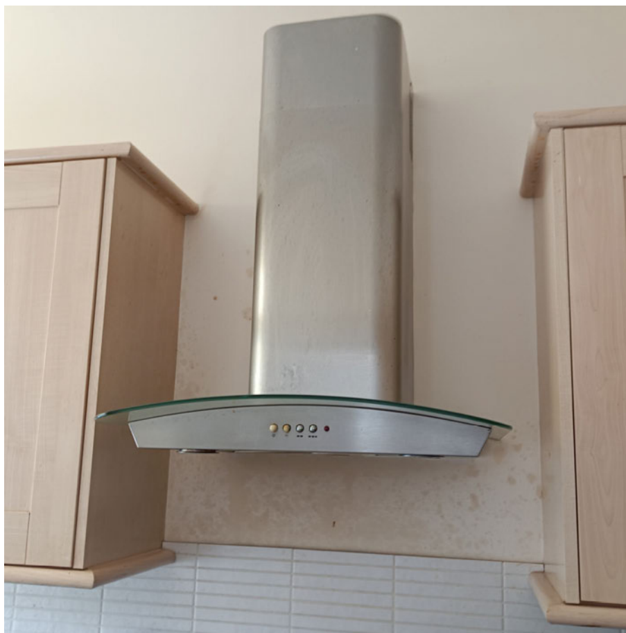
4 Inoperative kitchen extractor hood
