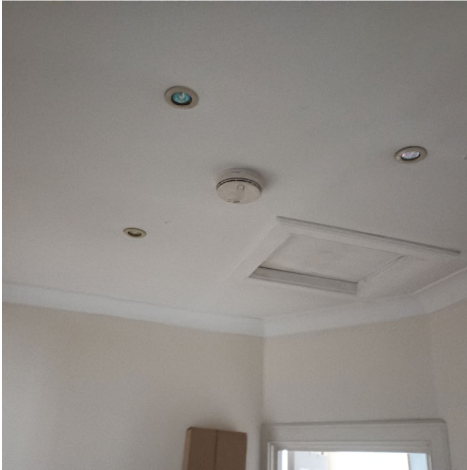
7 Defective smoke detector in the hallway
