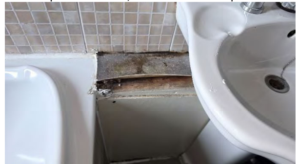
14 Damage to pipe boxing detail spanning between bath and wash basin.
