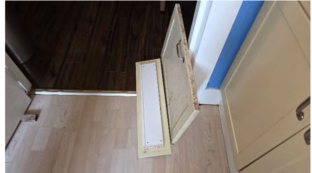
12 Example of retained, failed kitchen components.
