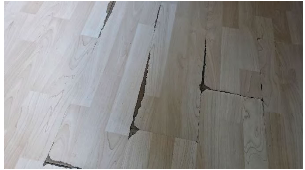
2 General view of laminate flooring deterioration to Kitchen flooring.
