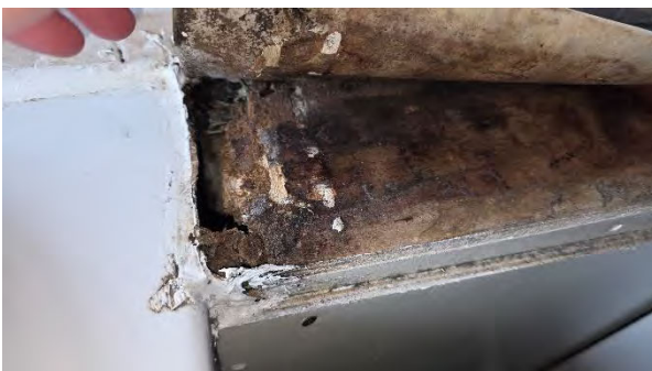
15 Close view of pipe boxing detail and timber decay arising from water escape from bath/shower area.
