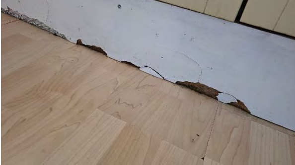
7 Damaged kitchen plinth/kickplate.
