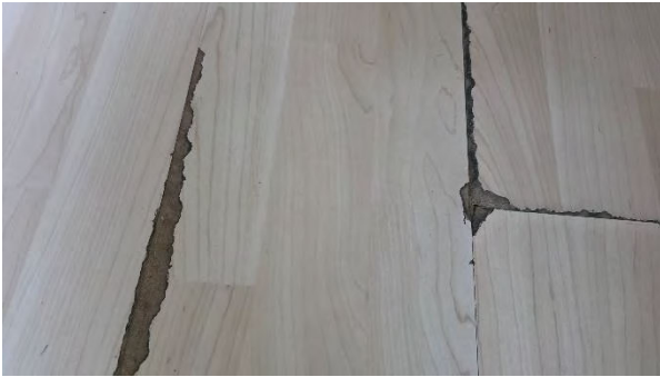
3 Close view of defective laminate flooring veneer within Kitchen.
