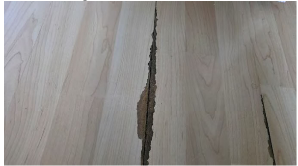
4 Close view of defective laminate flooring veneer within Kitchen.
