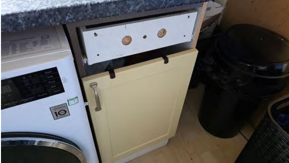
5 Missing drawer front to kitchen base unit.
