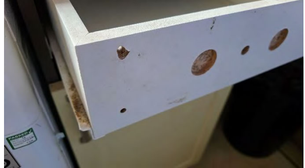
6 Close view of missing drawer front.
