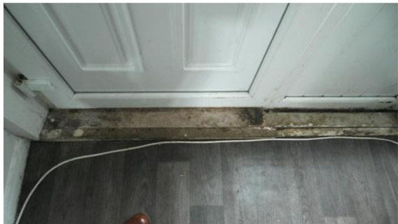
Photo 6 – Hall floor still damp behind front door
