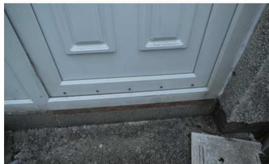
Photo 5 – Weather/drip bar still missing
