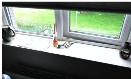
Photo 7 – Sill in front Bedroom remains loose
