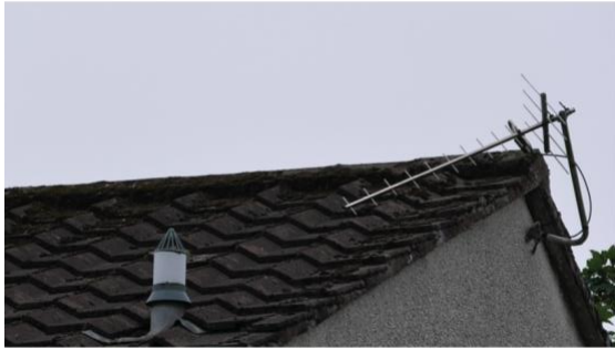
Photo 10 – No obvious signs of roof maintenance since original inspection on 03/03/2026
