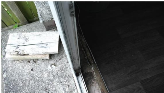
Photo 4 – Rubber seals still missing/broken
