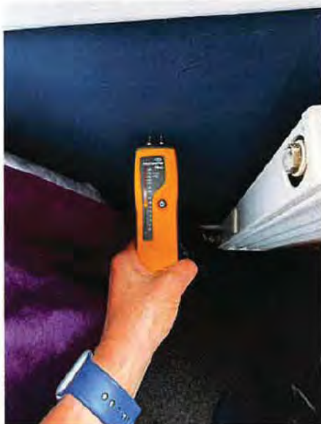
Photograph 16: Bedroom 3: Rear wall – damp meter showing slightly raised moisture levels
