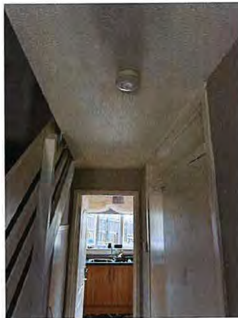
Photograph 5: Hallway: Smoke detector - interlinked and in working order
