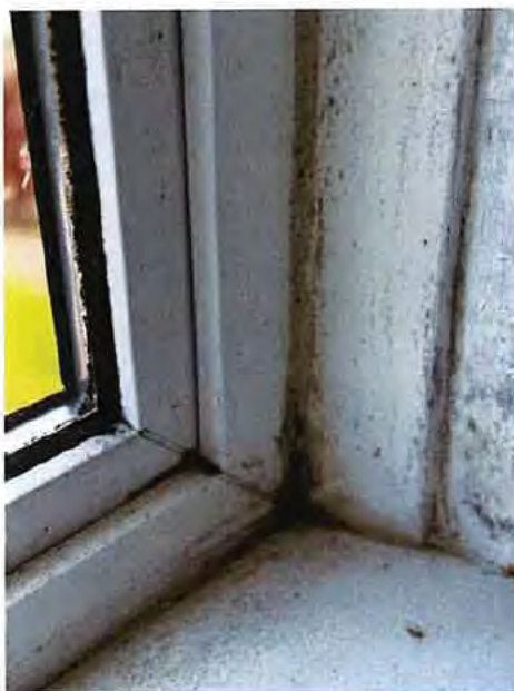
Photograph 17: Bedroom 3: Mould around window frame
