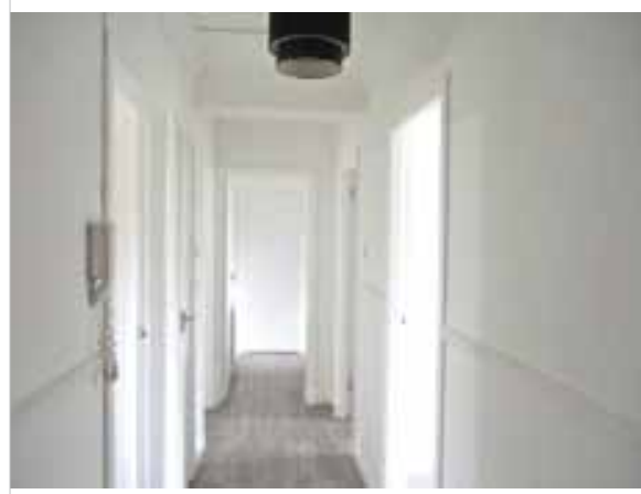
Hall - all floors level and door frames square
