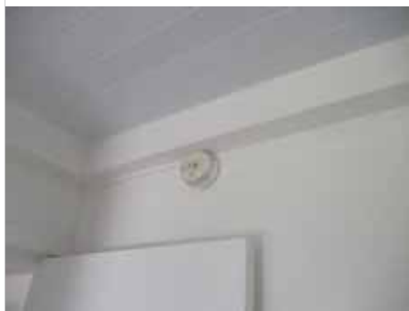
Kitchen - wall mounted heat detector
