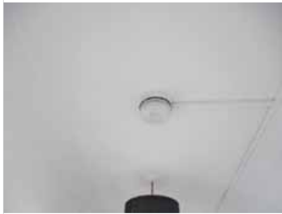
Hall - ceiling mounted smoke detector
