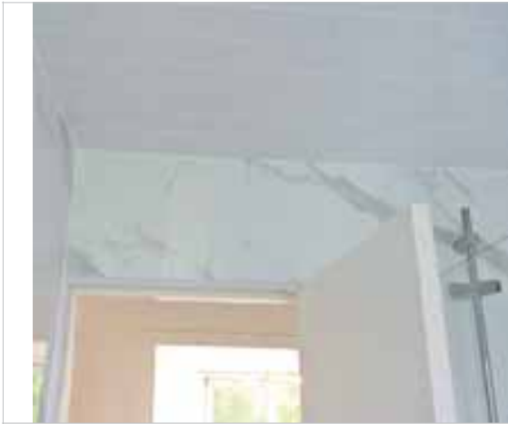
Bathroom - wall above door renewed, door frame square and floor level
