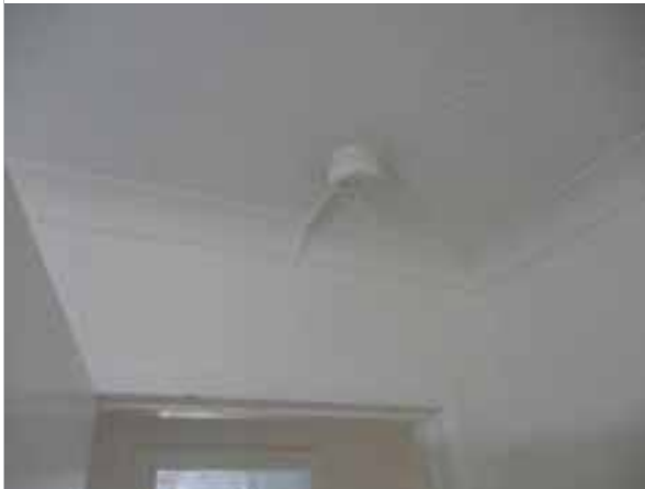
Living Room - ceiling mounted smoke detector
