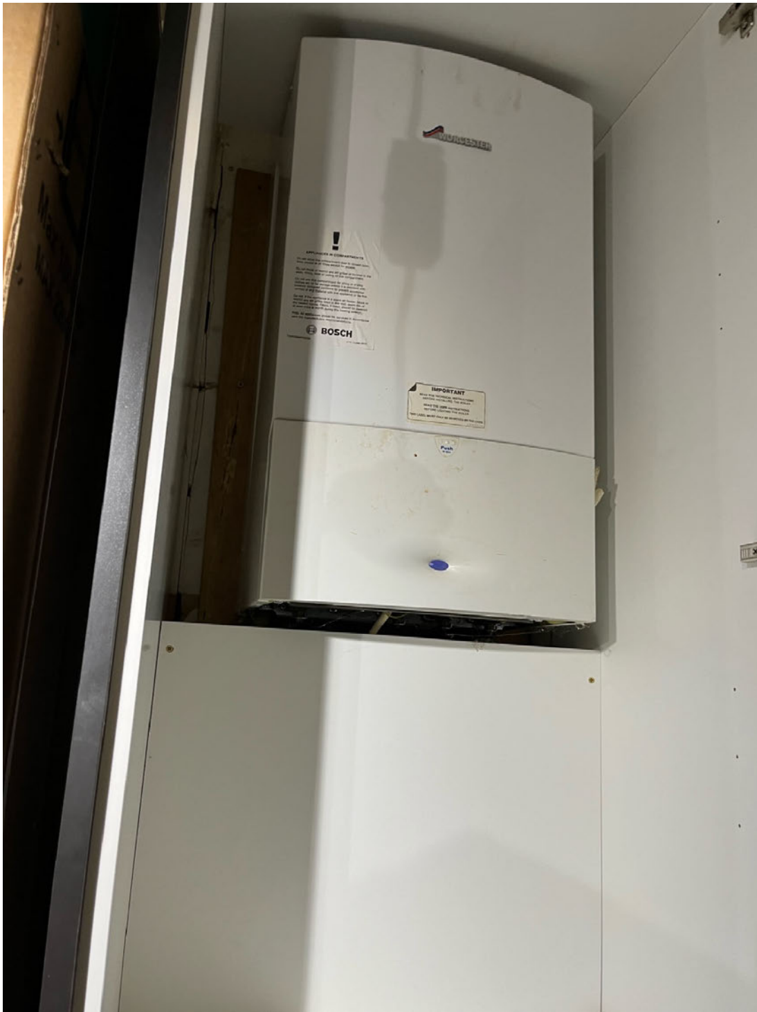
New Boiler cupboard
