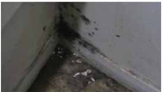
Photo 22 – Dampness and mould in hall cupboard
