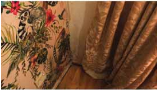
Photo 18 – Mould in main bedroom
