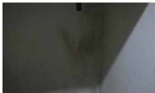
Photo 21 – Mould in main bedroom cupboard
