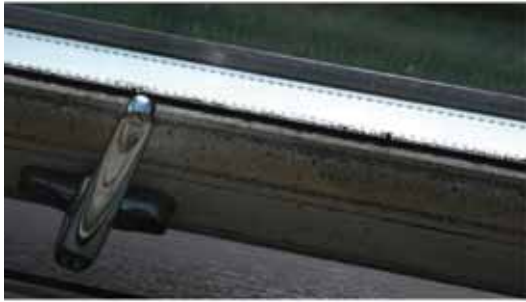
Photo 16 – Mould on living room window frame
