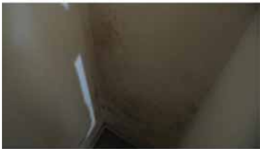
Photo 20 – Mould in main bedroom cupboard
