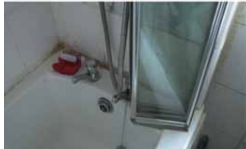
Photo 7 – Mouldy and failing sealant on bath
