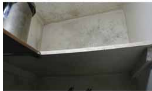
Photo 23 – Mould in hall cupboard
