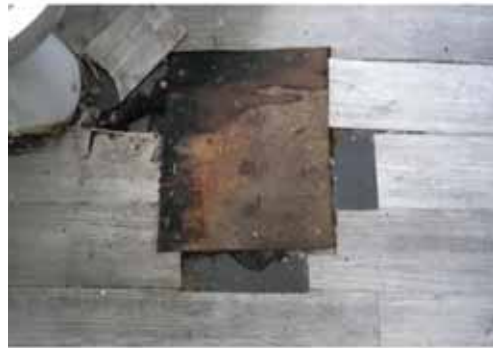
Photo 3 – Crude temporary fix
