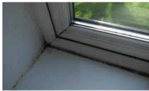
Photo 19 – Mould at main bedroom window
