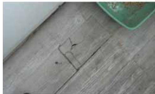
Photo 5 – Newly collapsed section of floor
