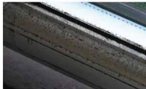
Photo 15 – Mould on living room window frame
