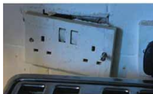
Photo 13 – Broken electrical double socket
