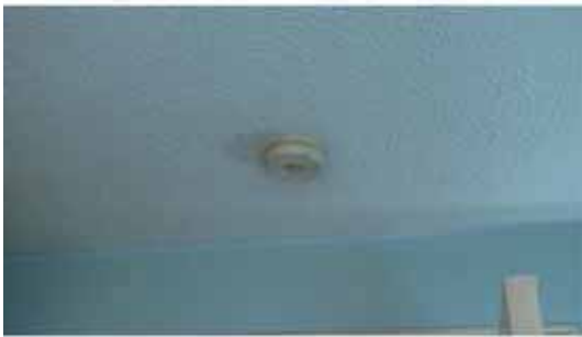
Photo 10 – Heat sensor on kitchen ceiling
