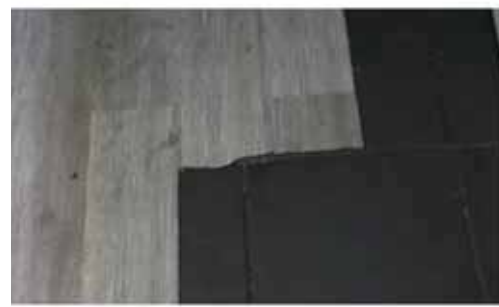
Photo 11 – Broken and missing laminate flooring
