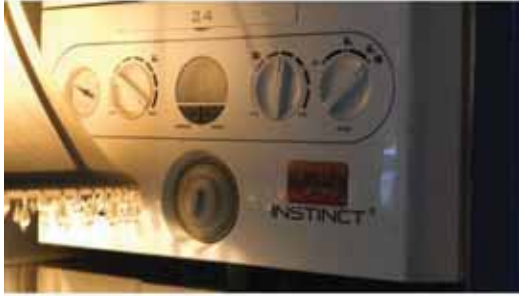
Photo 24 – Gas boiler in kitchen
