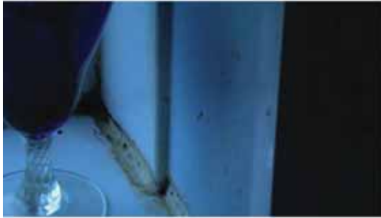
Photo 8 – Mould on sealant around kitchen window
