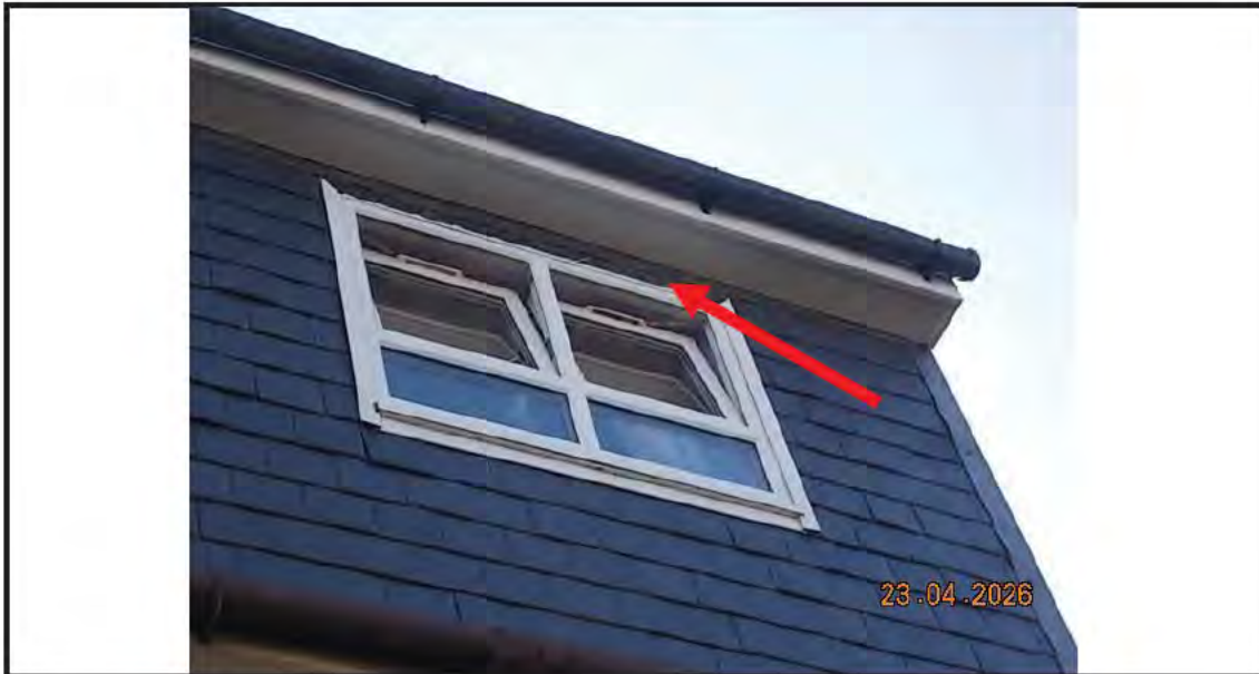
15. Missing trim (arrowed) above window in dormer to second floor rear bedroom
