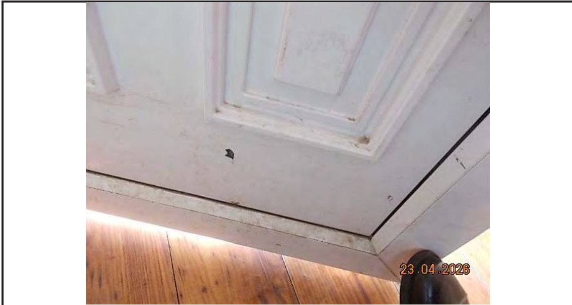
17. Front door inner face with damaged area
