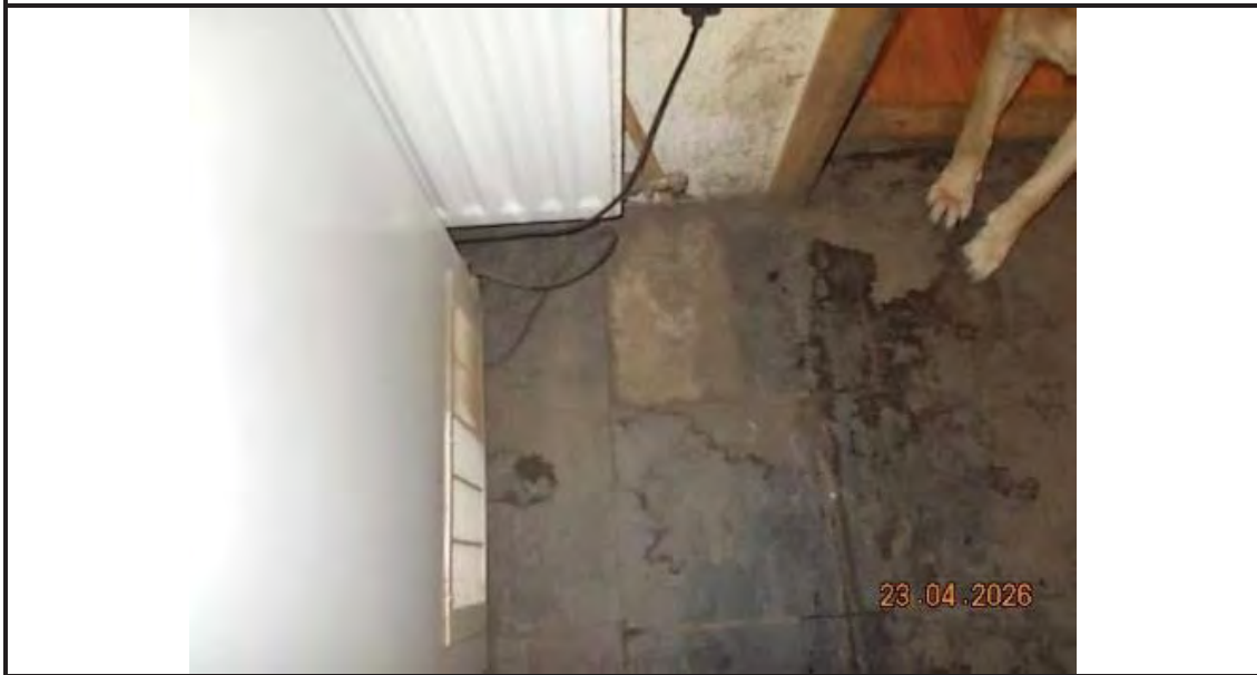
40. Gap to slate tile floor finish in Kitchen
