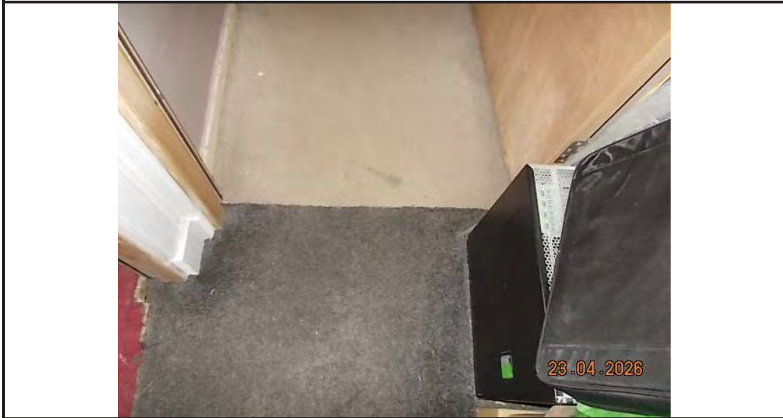
42. "Cover strip" missing at carpet joint, larger room, first floor at front of property to landing
