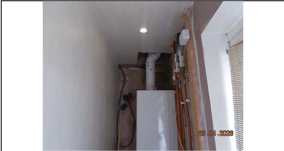
35. Area of displaced ceiling lining in smaller room, first floor at front of property
