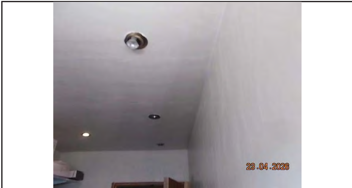
9. Lights not operational in Kitchen
