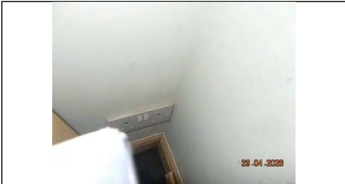
11. Socket outlet in rear bedroom at first floor level
