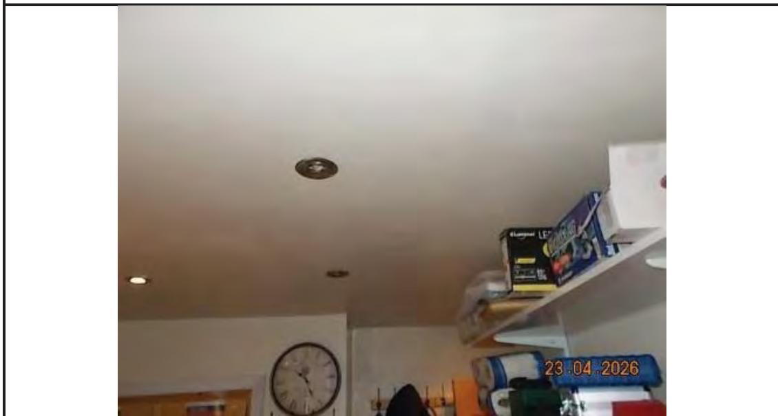
10. Lights not operational in smaller room, first floor at front of property
