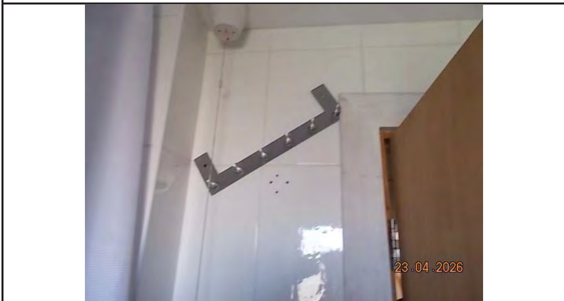
50. Coat hanger in Bathroom at First Floor level
