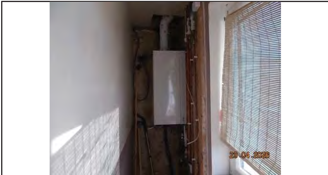
1. Boiler in smaller room, first floor at front of property
