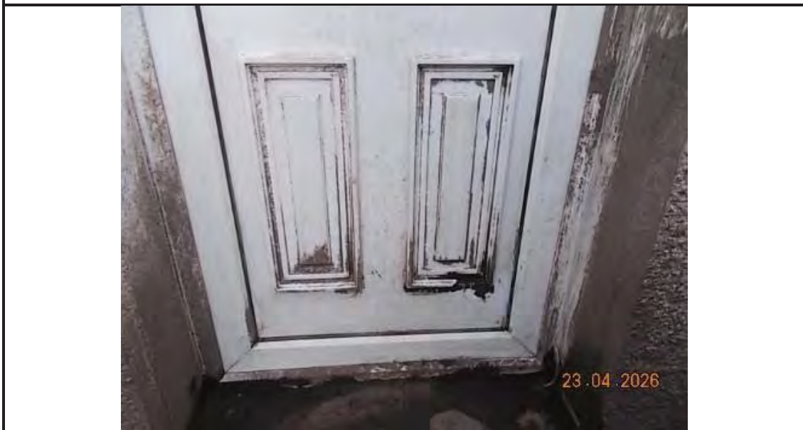
18. Rear door outer face with damaged area to lower right panel
