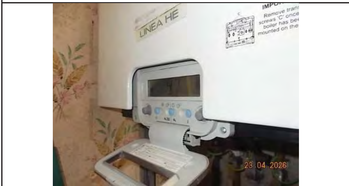
2. Boiler in smaller room, first floor at front of property
