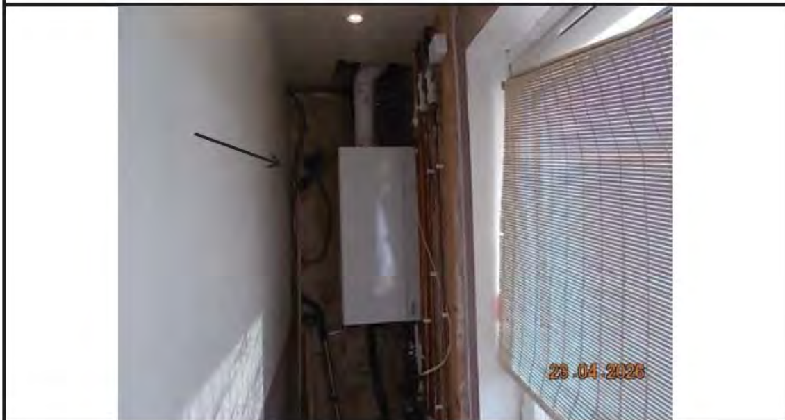
14. Cable connectors on wall arrowed
