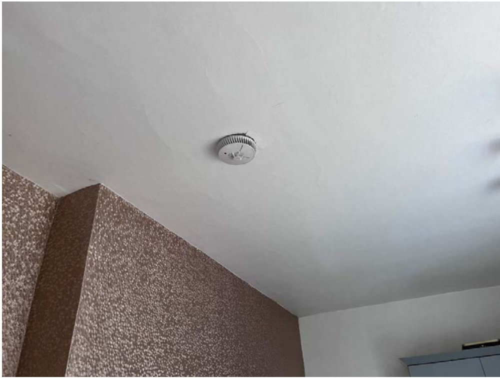
Smoke detector on Kitchen ceiling.
