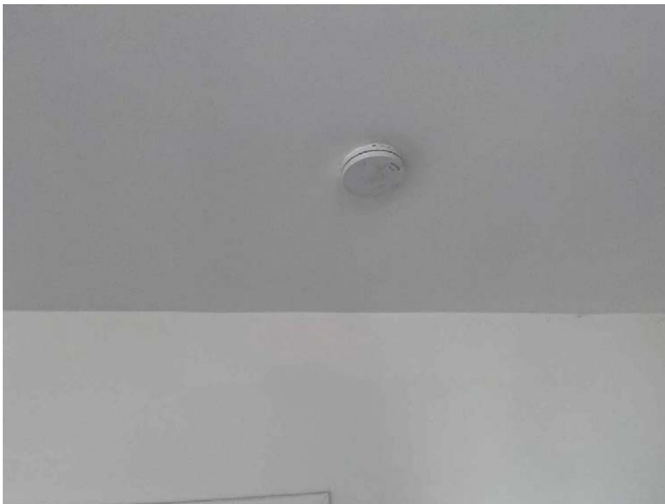
Smoke detector on Living Room ceiling.
