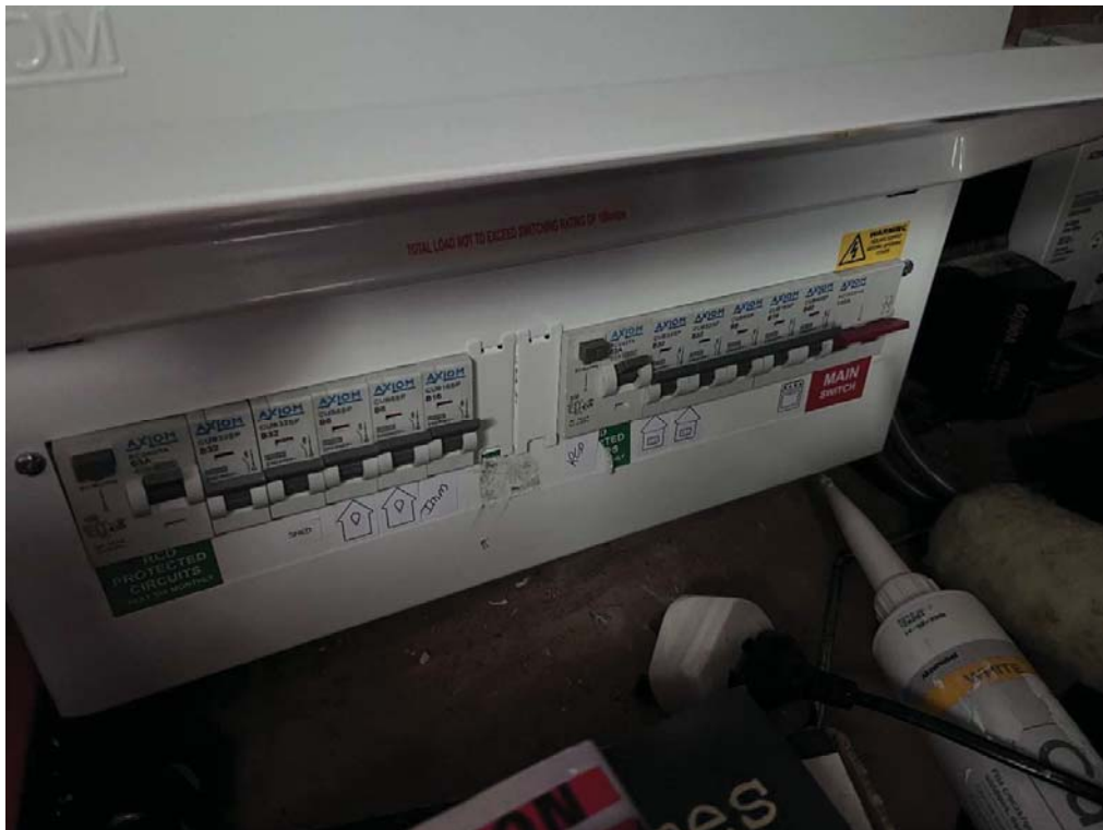
Fusebox in Kitchen cupboard.
