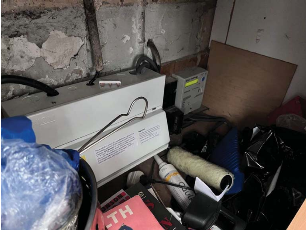
Fusebox and electric meter in Kitchen cupboard.
