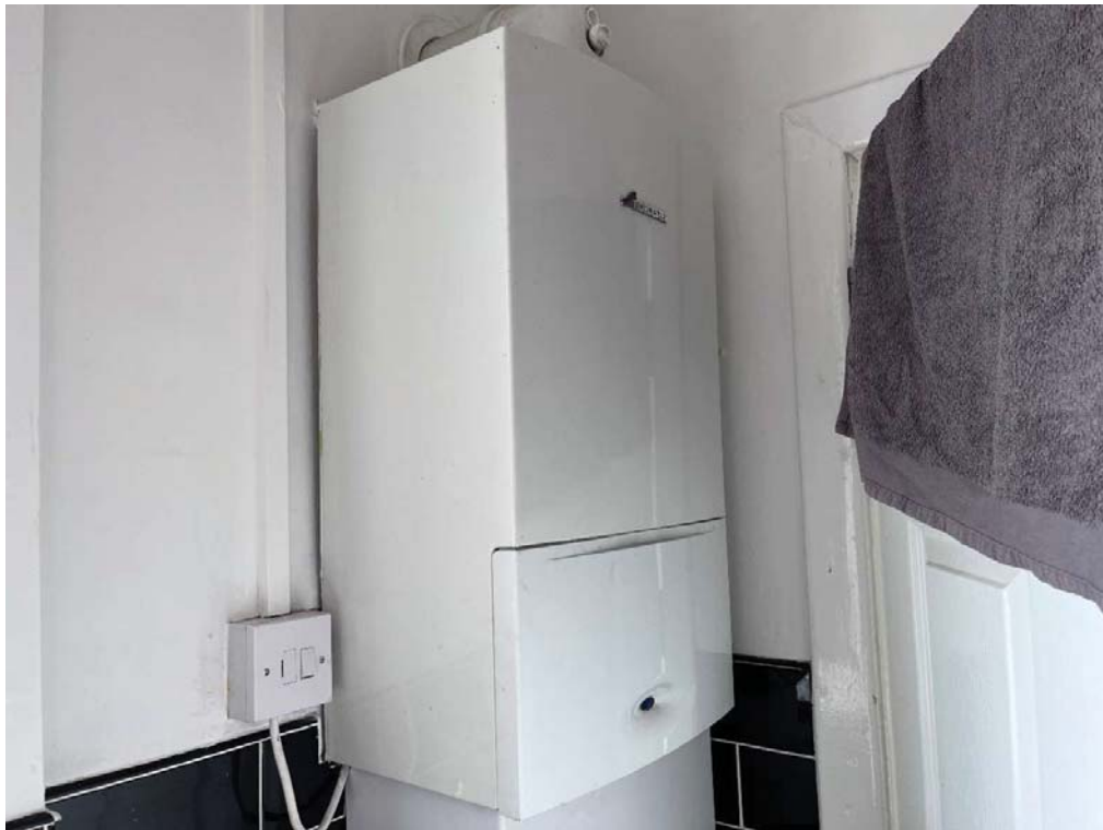
Central Heating Boiler in Kitchen.
