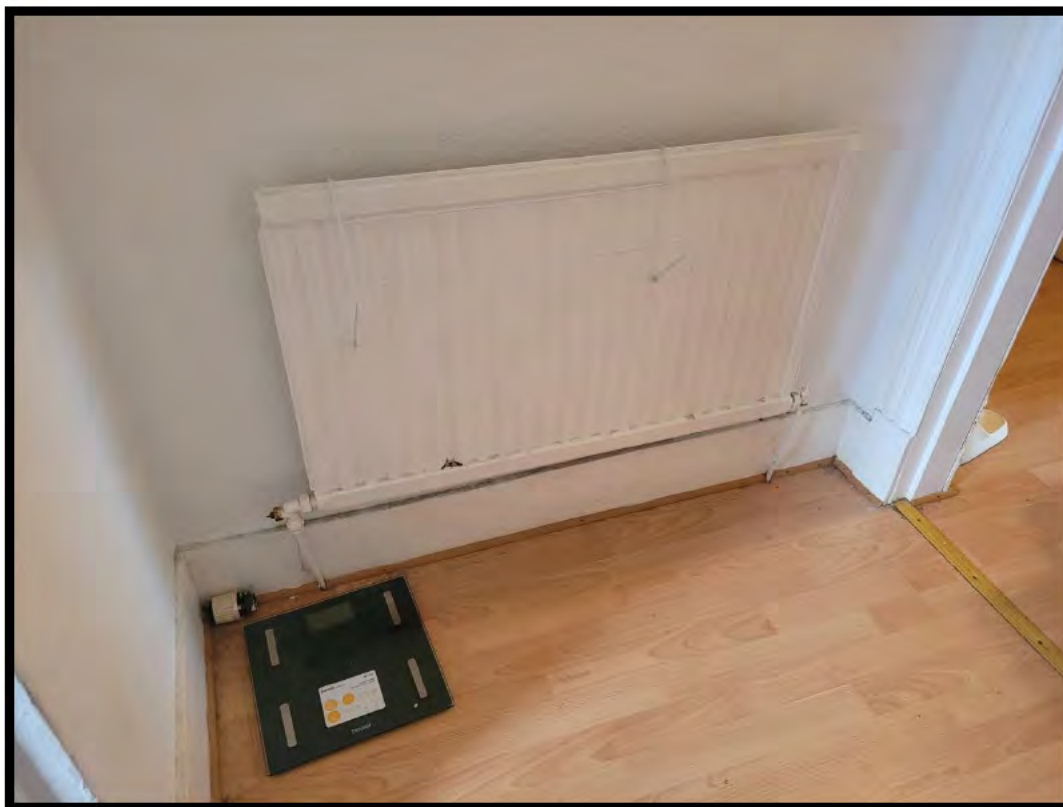
Photograph 10 Bedroom: Radiator with detached TRV.
