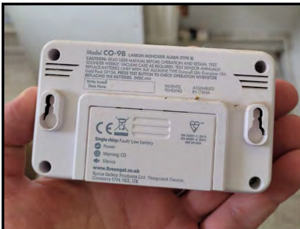
Photograph 3 Kitchen : CO Alarm. Installation date blank, removable battery type
