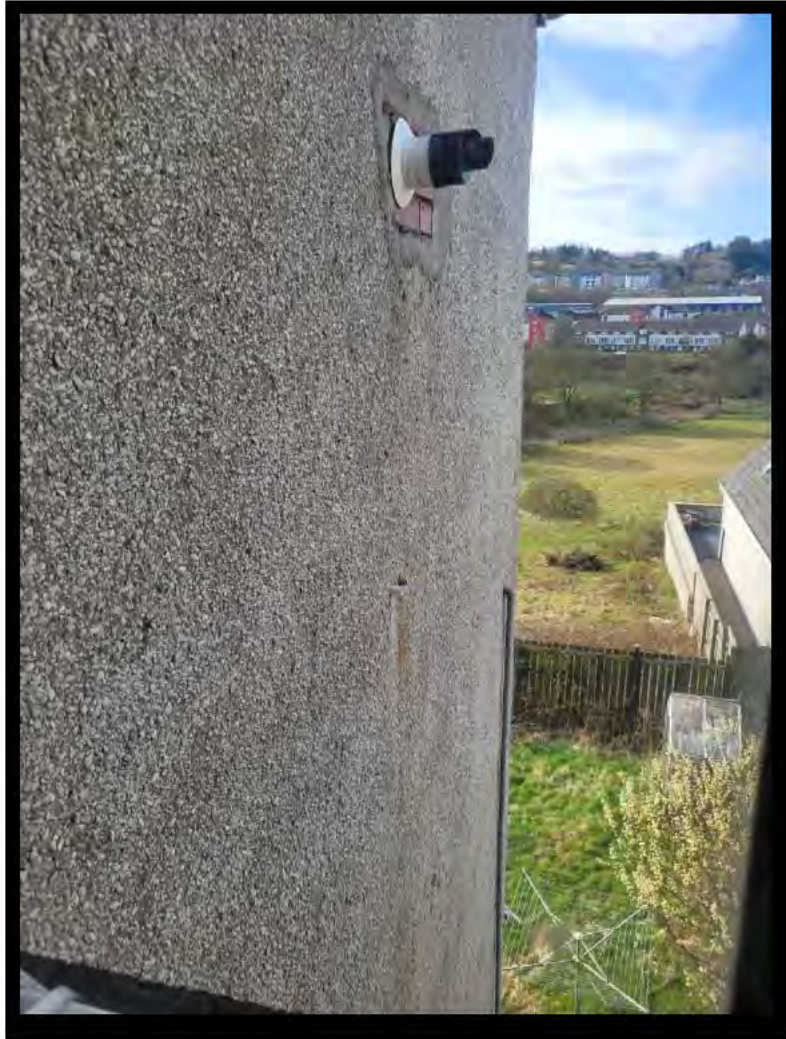
Photograph 5 Kitchen wall external: Condensate drain pipe section missing.
