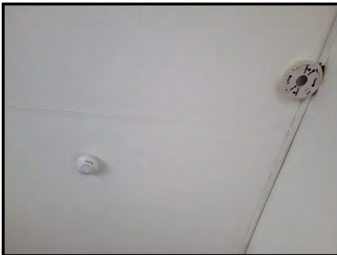
Photograph 7 Lounge: Smoke alarm and remains of previous installation.
