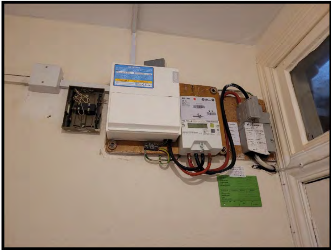
Photograph 8 Hallway: Electrical installation.
