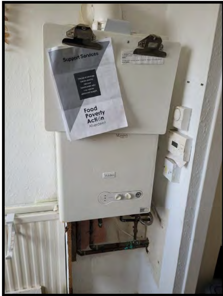
Photograph 4 Kitchen: Central heating boiler. Not operational, pressure gauge reading zero.
