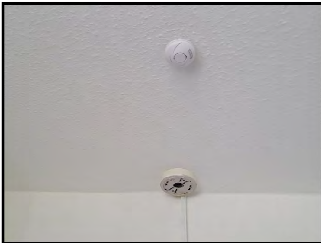
Photograph 6 Kitchen: Heat alarm and remains of previous installation.
