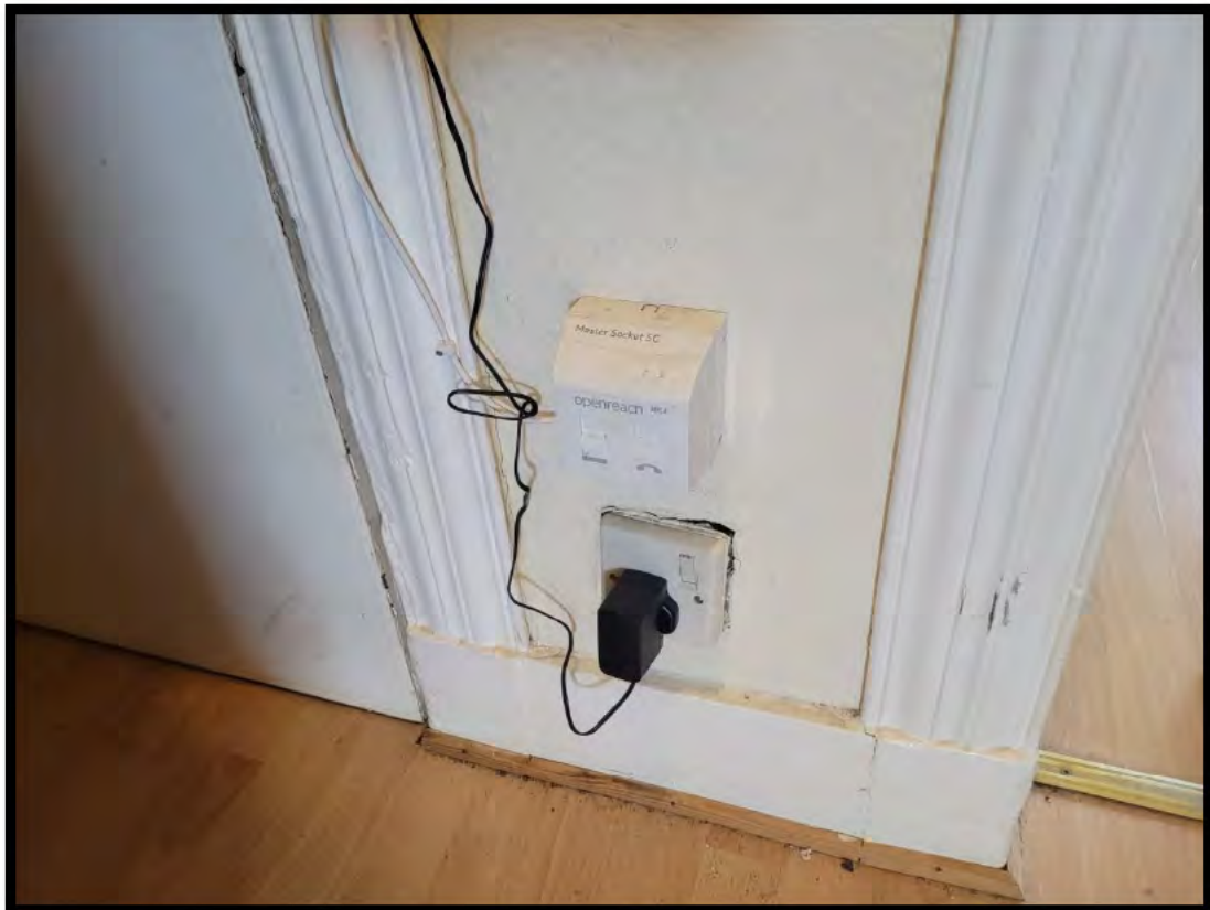
Photograph 9 Hallway: Loose electrical socket.
