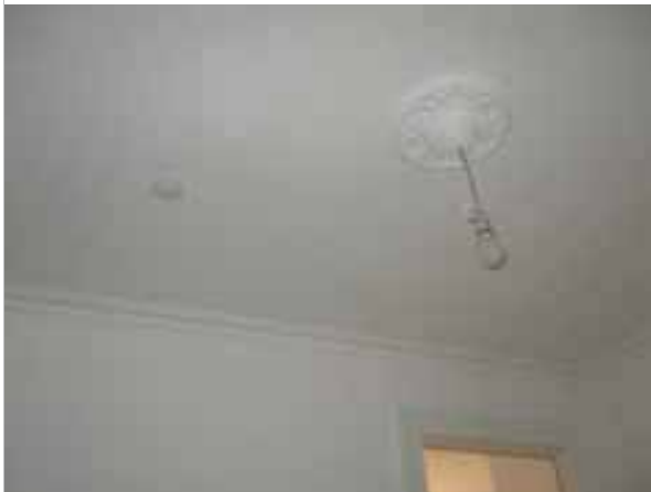
Hall - ceiling mounted smoke detector
