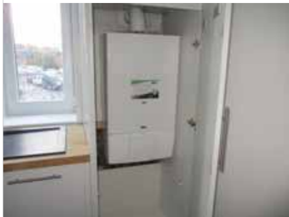
Kitchen - gas boiler housed in cupboard - no CO detector
