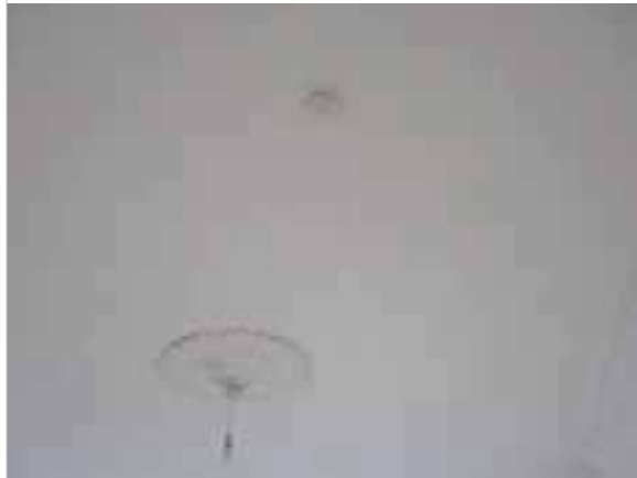
Living Room - ceiling mounted smoke detector
