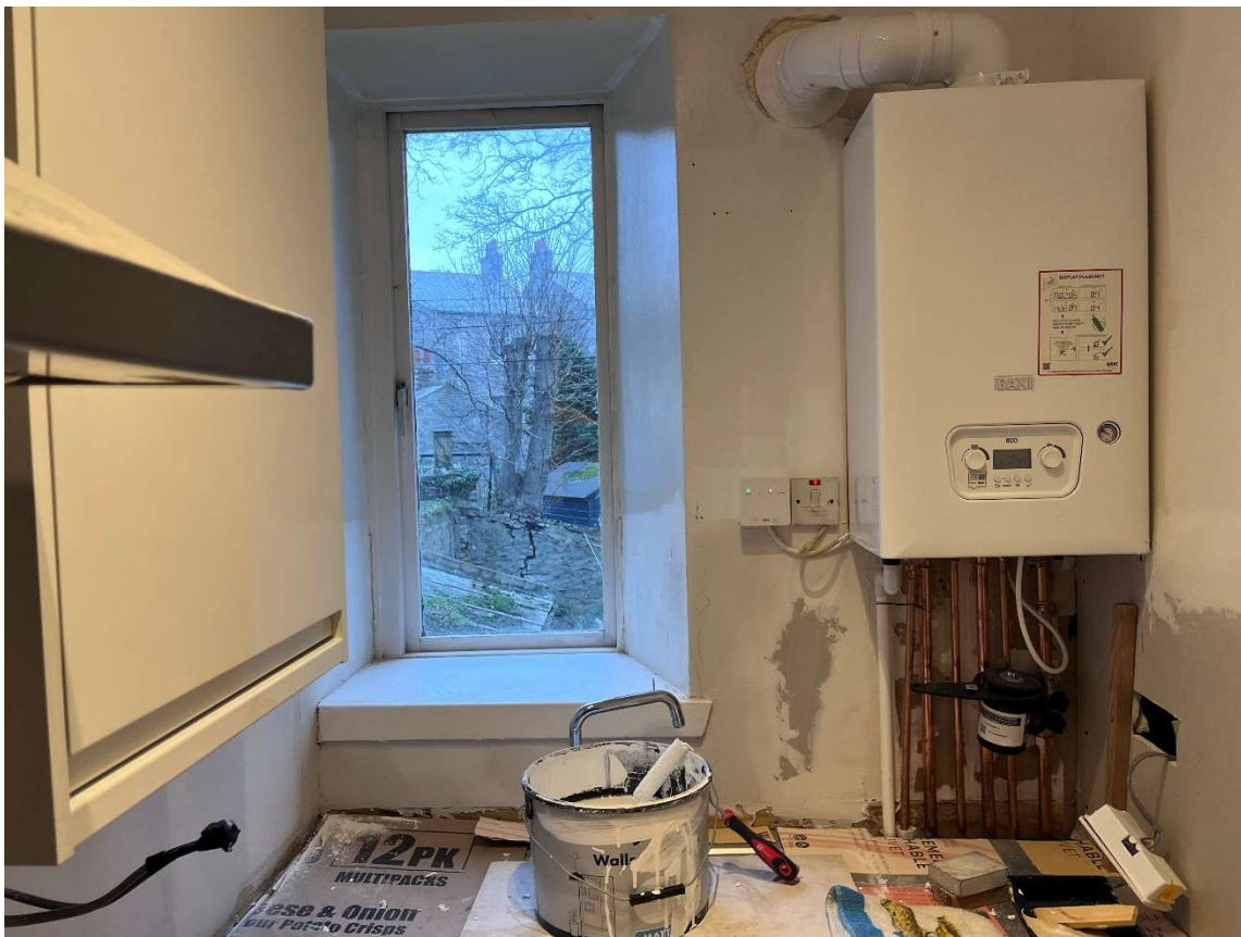
General view of Kitchen and replacement central heating boiler.
