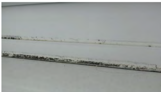
Photo 14 – Mould on skirtings
