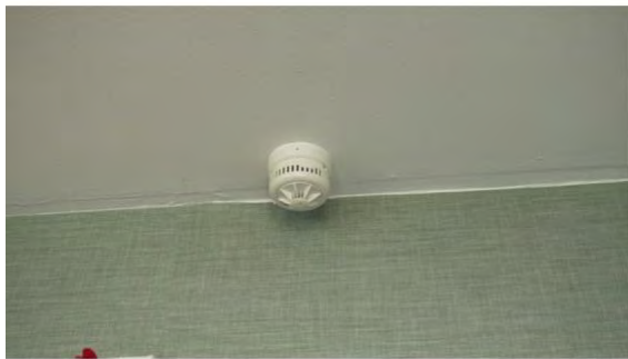
Photo 18 – Heat sensor in Kitchen
