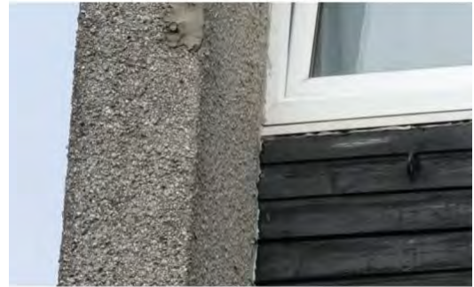
Photo 11 – Poorly sealed cladding/render joint
