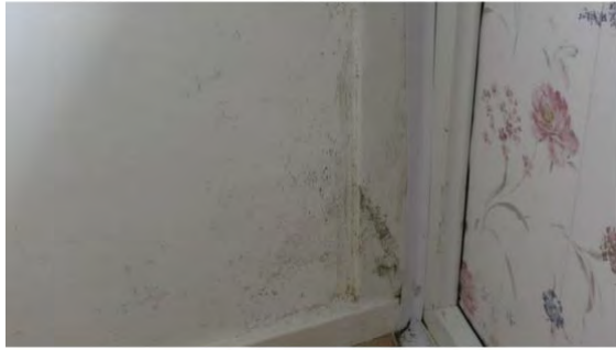
Photo 16 – Mould and dampness issues
