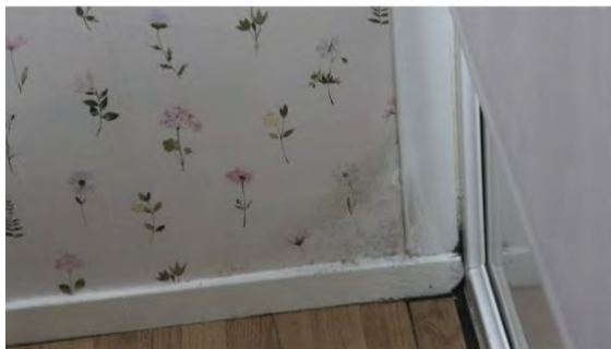
Photo 12 – Dampness and mould issues
