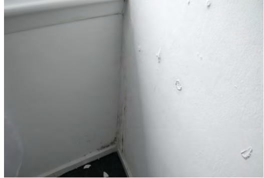
Photo 17 – Severely damp section of L/R wall
