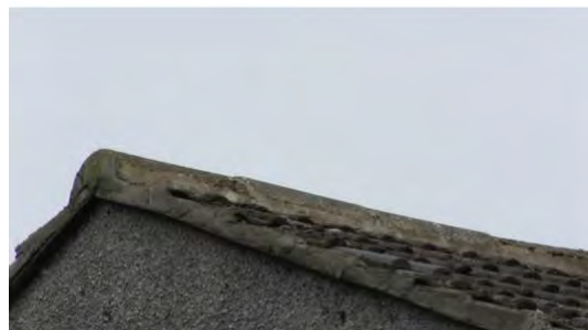
Photo 23 – Crude mortar repairs to ridge + verge
