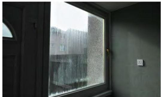
Photo 7 – Failed sealed glazing unit in Kitchen
