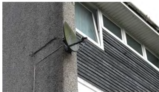
Photo 21 – Cracked render behind dish
