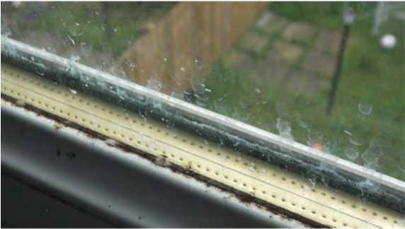
Photo 4 – Failed sealed glazing unit in Bedroom
