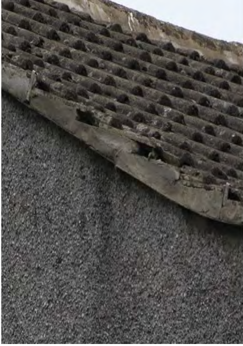
Photo 24 – Missing mortar + visible holes at verge
