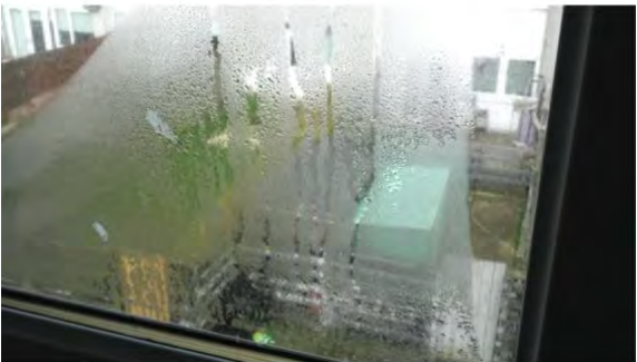
Photo 6 – Failed sealed glazing unit in Living room
