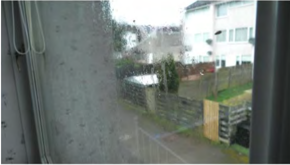
Photo 2 – Failed sealed glazing unit in Bedroom
