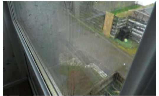
Photo 5 – Failed sealed glazing unit in Bedroom
