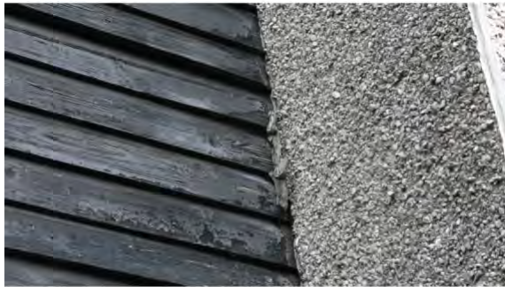
Photo 10 – Cladding/Render joint exposed to rain
