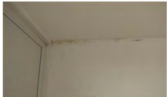
Photo 13 – Mould on ceiling
