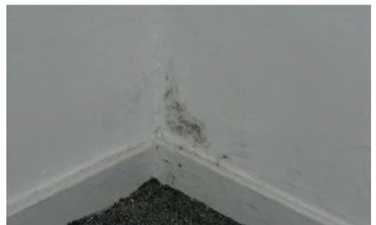
Photo 15 – Mould and dampness issues
