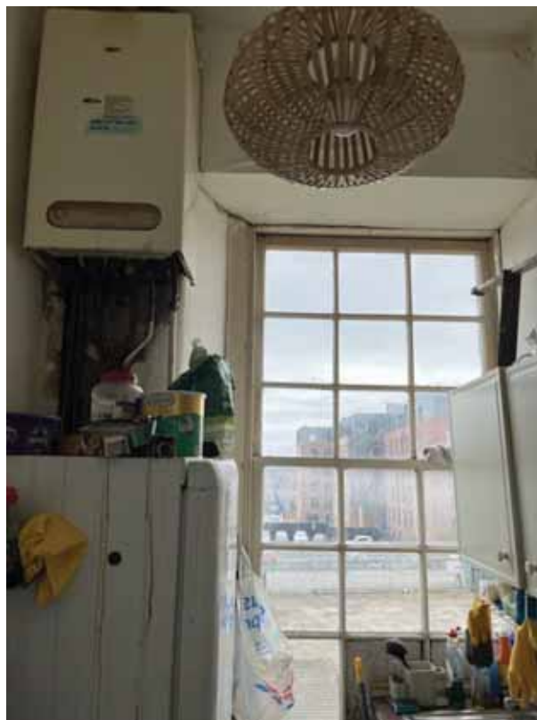
Kitchen window and boiler
