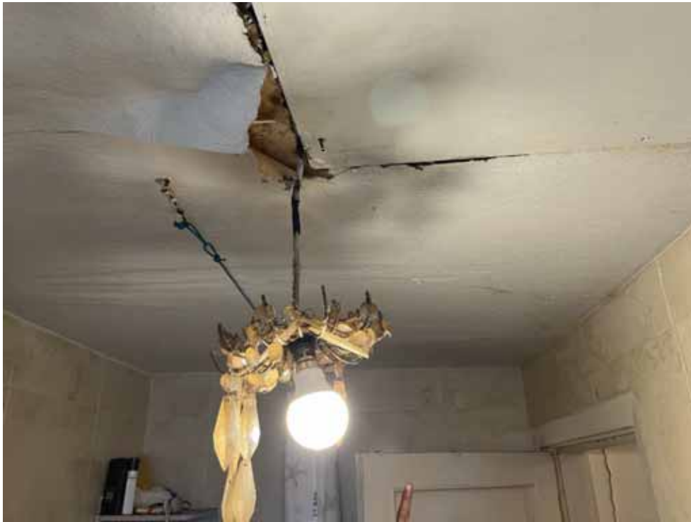
Light fitting in the bathroom
