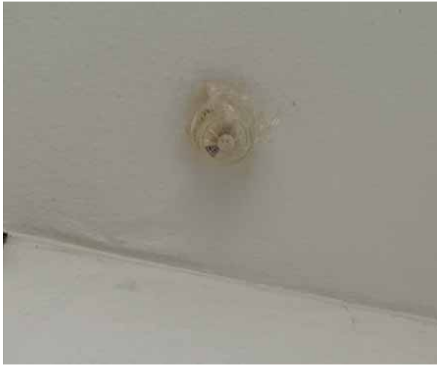
Heat detector in the kitchen
