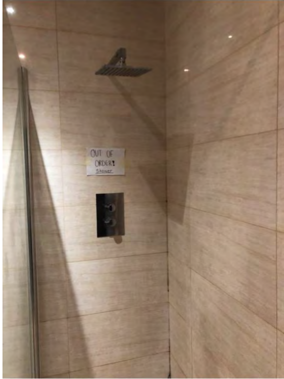
Photo 2 – Main ensuite + failed sealant on tiles
