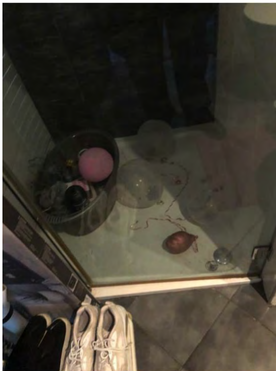
Photo 20 – 2 nd ensuite shower enclosure leaking
