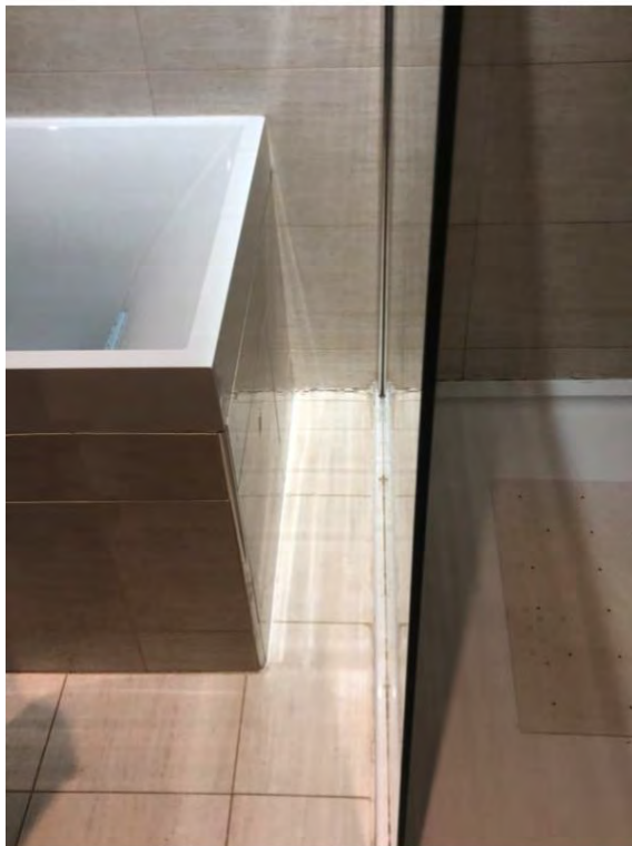
Photo 4 – Failed sealant between bath and shower
