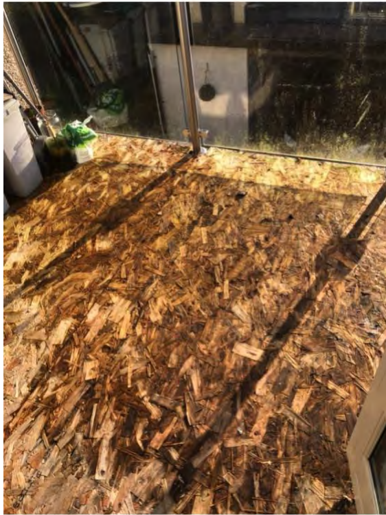
Photo 18 – Temporary fix to balcony floor hole
