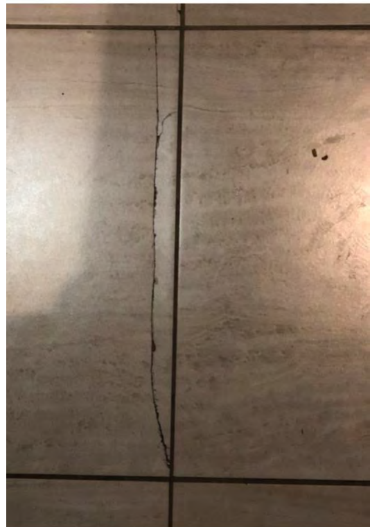
Photo 5 – Cracked main ensuite floor tile
