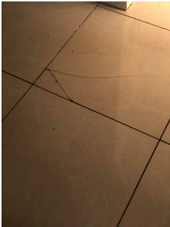
Photo 16 – Broken floor tiles in kitchen
