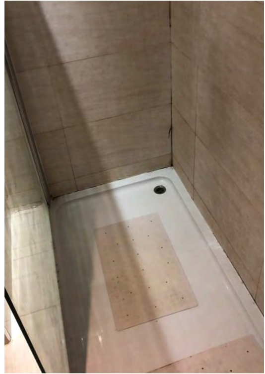
Photo 3 – Failed sealant around shower tray
