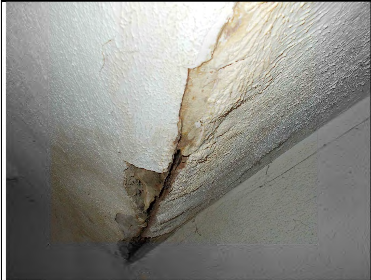
9. Stair to Attic Level. Water damage reported indicative of water penetration at valley gutter.
