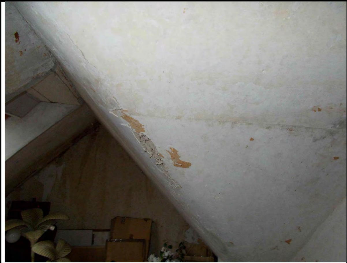
10. Attic storeroom to rear. Indicated previous water penetration from valley gutter.
