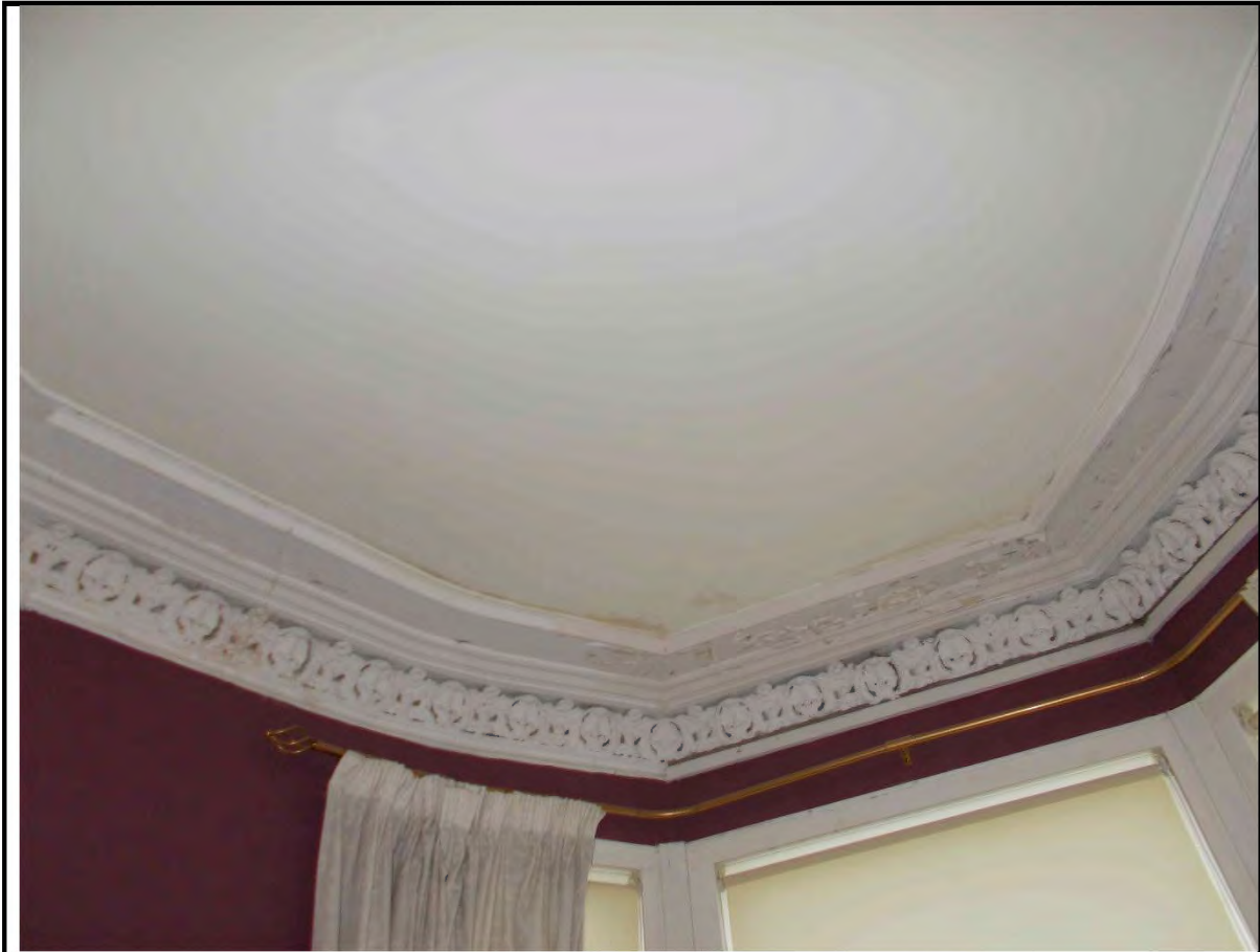
5. Front Bedroom Bay Window ceiling with signs of previous water penetration reported as not currently active.
