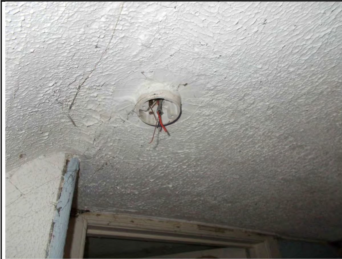
21. Exposed electrical wiring on Attic Level Stair Landing ceiling.
