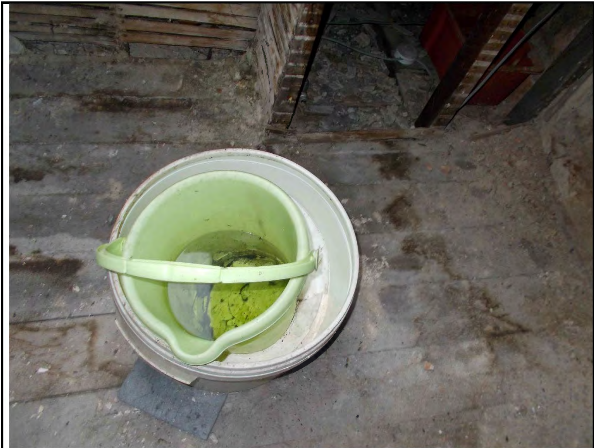
14. Water collected in bucket below Velux window above Dressing Room below.
