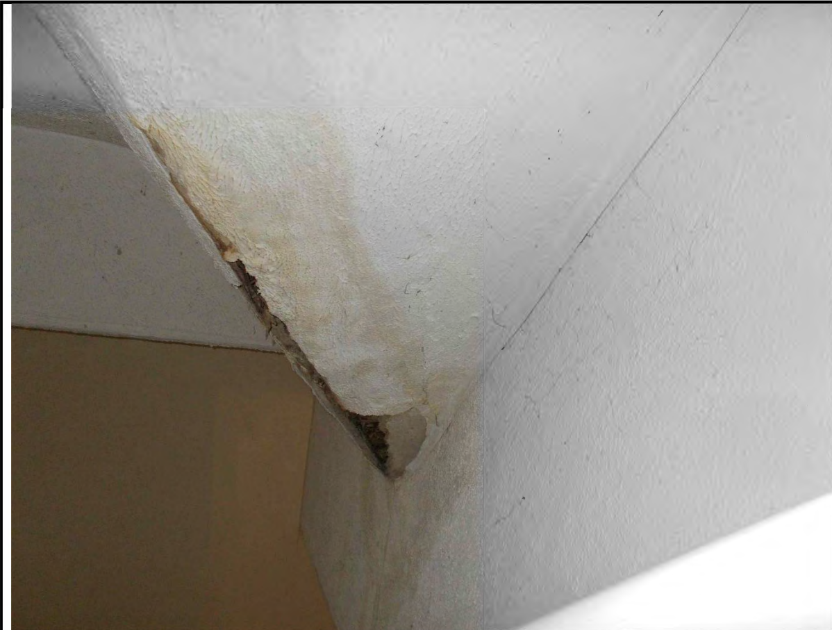
8. Stair to Attic Level. Water damage reported indicative of water penetration at valley gutter.
