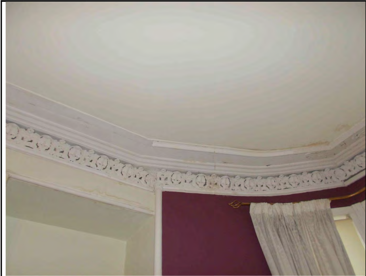
6. Front Bedroom Bay Window ceiling with signs of previous water penetration reported as not currently active.
