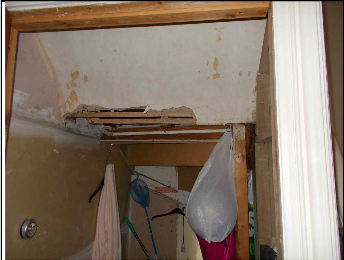
7. Cupboard below stair to Attic Level. Plasterwork damaged reportedly following water penetration.
