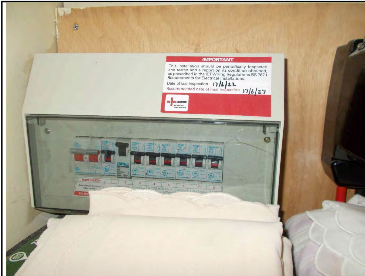
20. Electrical Consumer Control Unit
