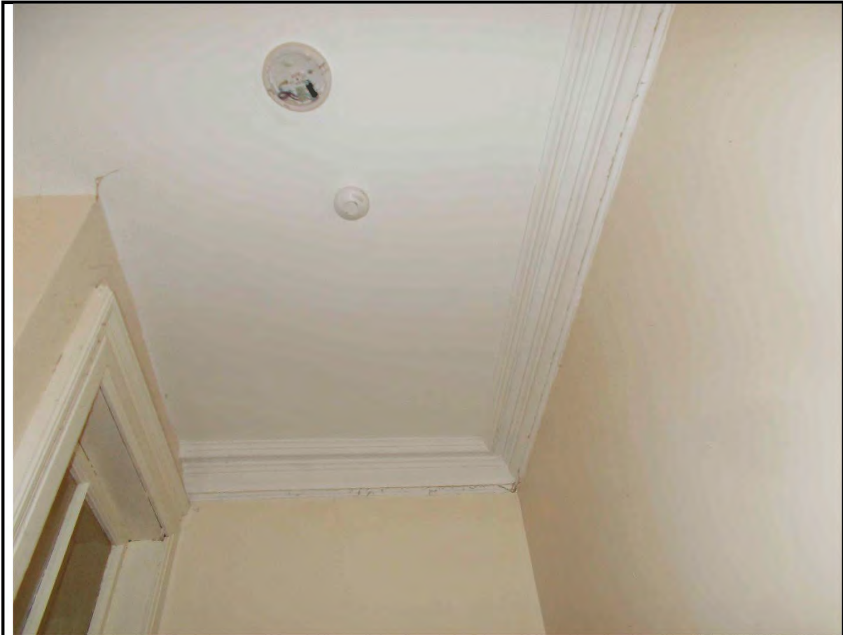
22. Base plate for removed Smoke alarm in Hallway at Kitchen door.
