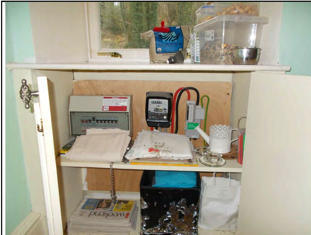
19. Electrical Consumer Control Unit
