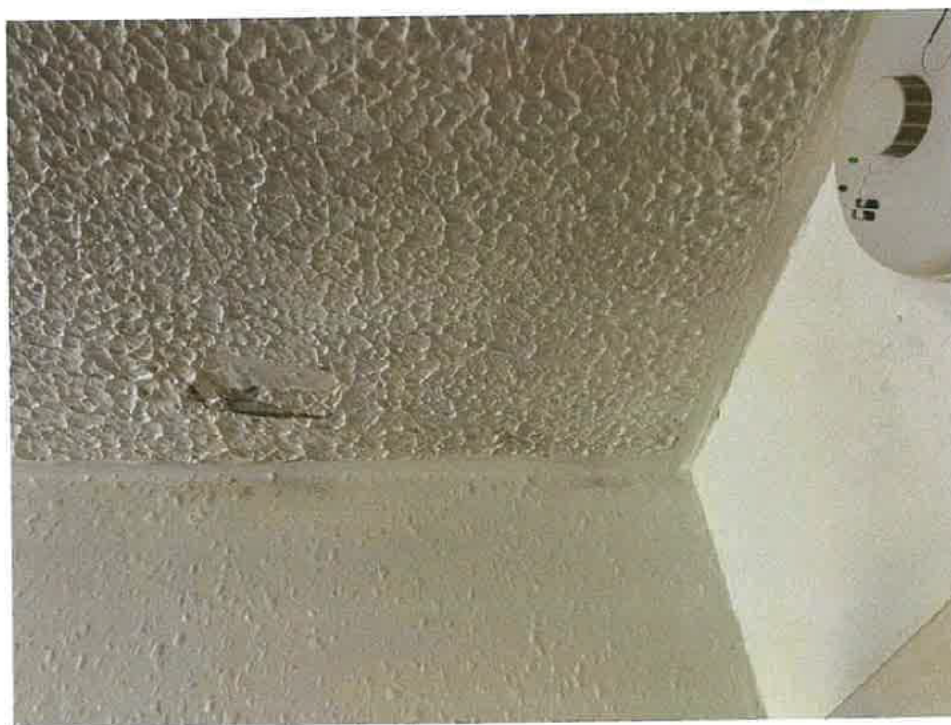
Damp staining/plaster damage to ceiling in Kitchen.
