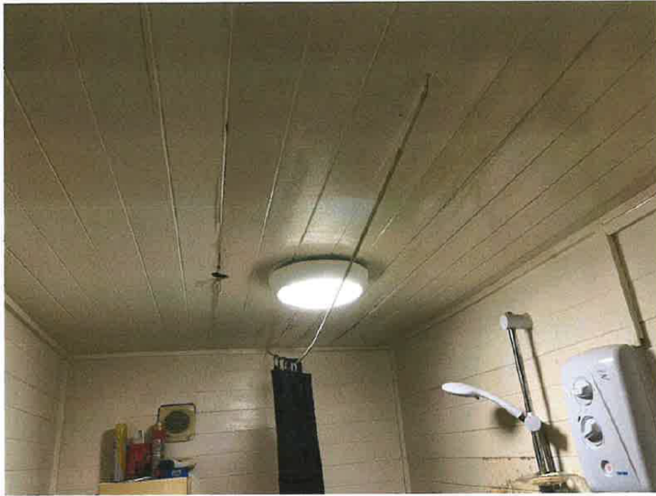
Damp staining/condensation mould to ceiling in Bathroom.
