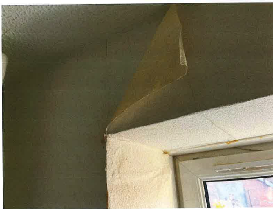
Damp staining on upper wall/ceiling of Kitchen.
