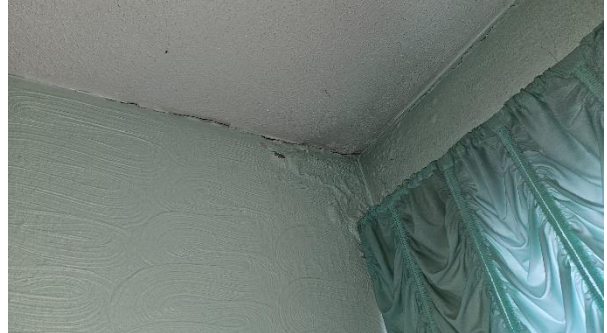
6 Bedroom 2 – blistered paintwork above window area to corner of room.
