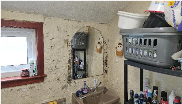
9 Bathroom – general heavy mould contamination evident throughout.
