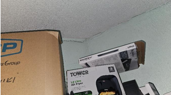
5 Bedroom 2 – minor cracking towards ceiling junctions.
