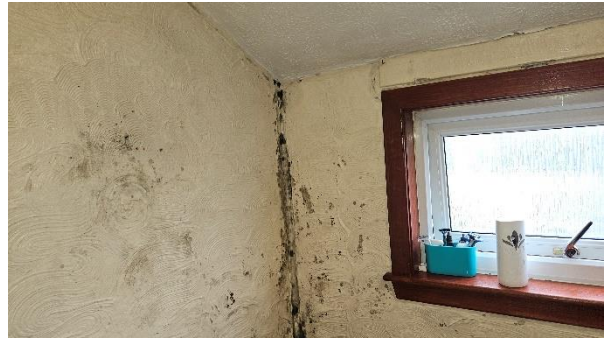
10 Bathroom – general heavy mould contamination evident throughout.
