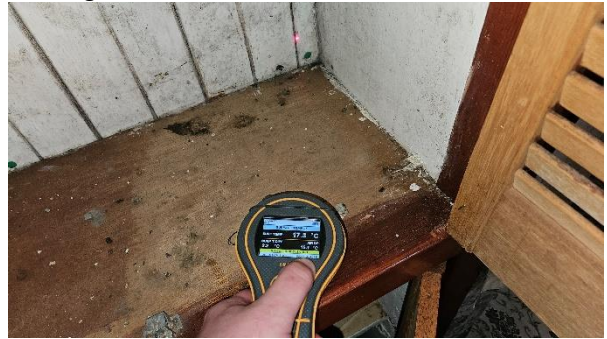
4 Risk of Condensation within Bedroom 1 cupboard.
