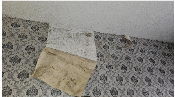
2 Areas of peeling wallpaper within Bedroom 1 and mould growth.
