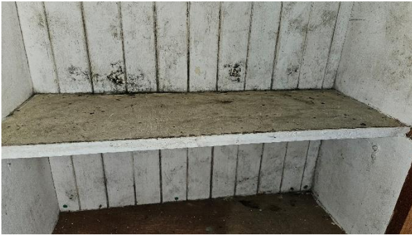
3 Mould growth within louvred cupboard within Bedroom 1.
