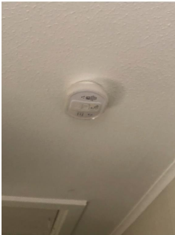
Photo 8 – Smoke detector on Landing
