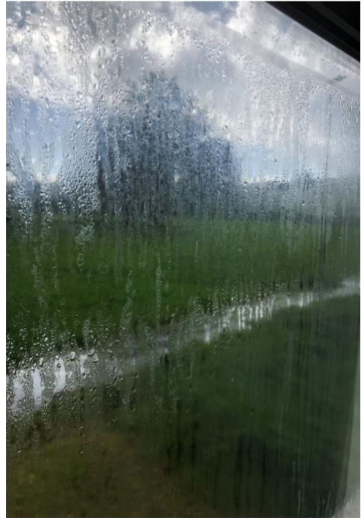
Photo 3 – Failed Lounge window glazing
