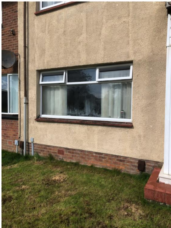
Photo 4 – Fogged glazing cavity in Lounge window
