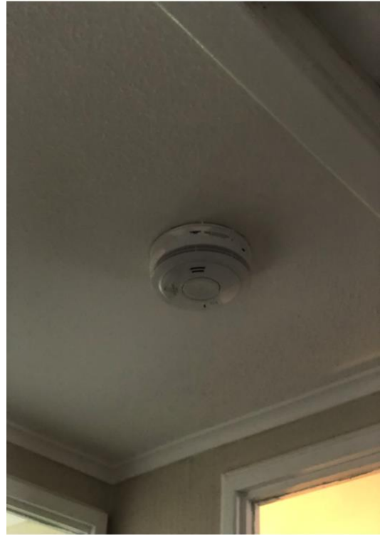
Photo 7 – Heat detector in kitchen
