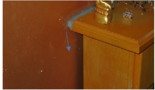
Photo 3 – Crudely attached fire surround and gap
