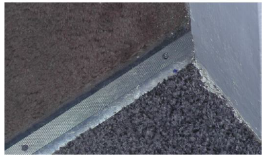
Photo 5 – Raised screwhead on Bedroom threshold
