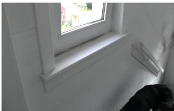
Photo 8 – Mould at Landing Head window
