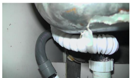
Photo 7 – Kitchen sink overflow now in place
