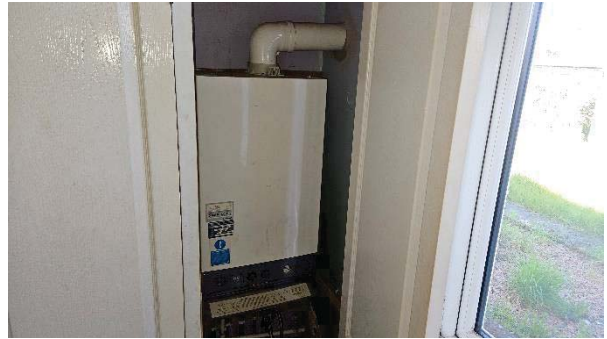
18 Gas fired boiler.
