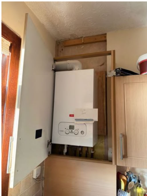
Photograph 5: Kitchen: Gas boiler in cupboard
