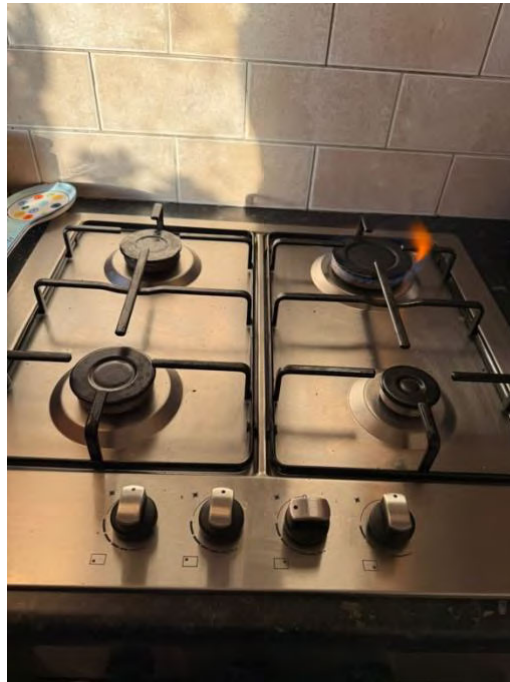
Photograph 2: Kitchen: Gas hob (working)
