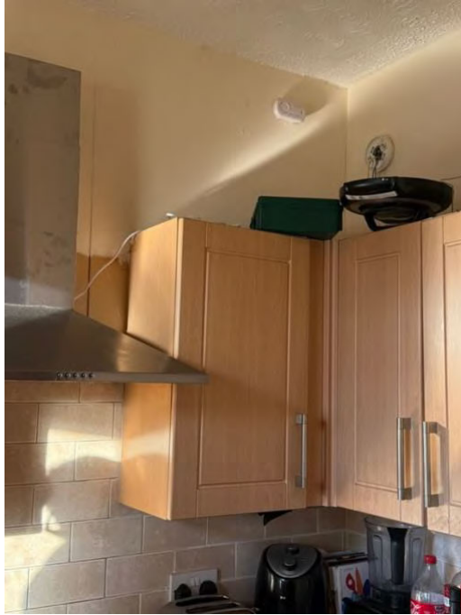
Photograph 6: Kitchen: Carbon monoxide detector
