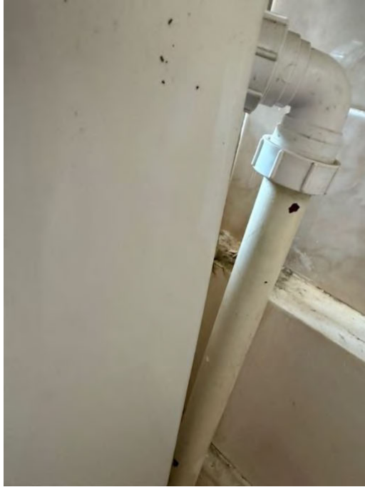
Photograph 12: Bathroom: Sink waste pipe
