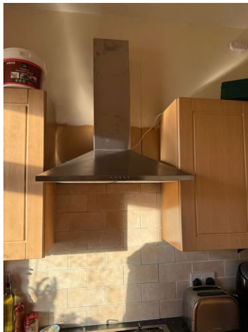
Photograph 3: Kitchen: Extractor hood
