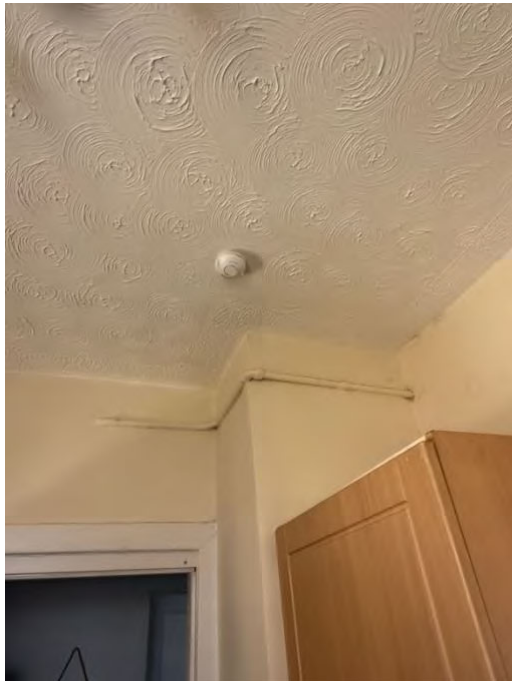
Photograph 7: Kitchen: Heat detector (not working)
