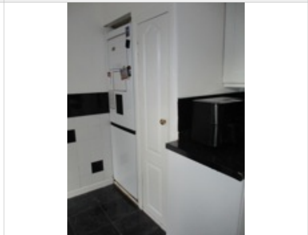
Kitchen - large cupboard - door is hard to open and close properly/ill fitting and handle loose
