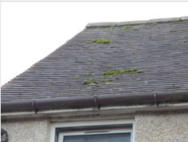
Front elevation - some roof tiles showing signs of deterioration/dislodged and patches of moss
