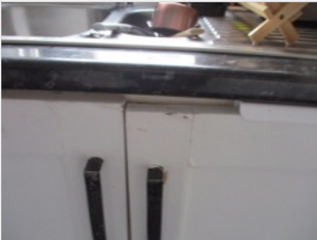
Kitchen - double base unit under sink - right side door misaligned
