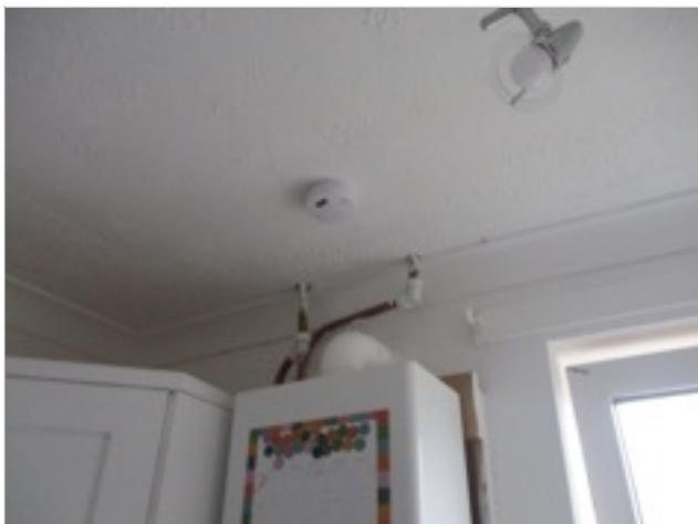
Kitchen - ceiling mounted carbon monoxide detector - appears not to be sited between 1 and 3 metres from the appliance (observation)
