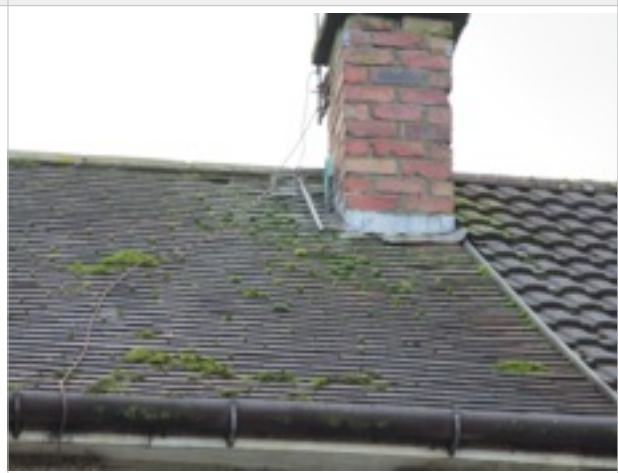
Front elevation - some roof tiles showing signs of deterioration/dislodged and patches of moss
