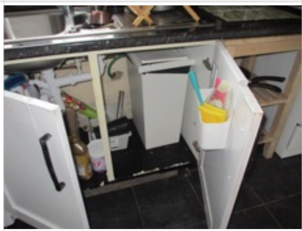
Kitchen - double base unit under sink - damage to base of interior right side unit (tenant has temporarily removed kick plates for cleaning purposes)
