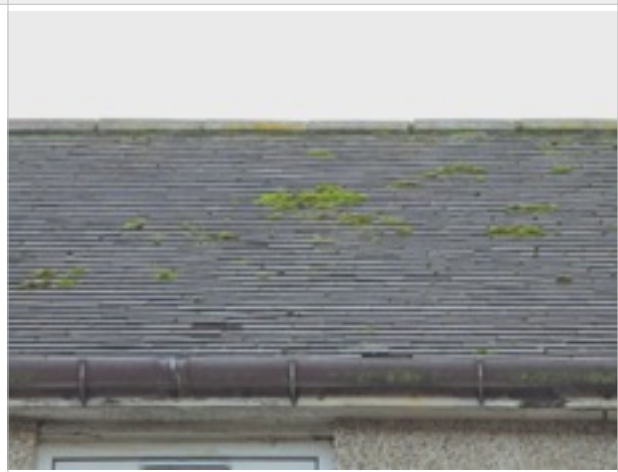
Front elevation - some roof tiles showing signs of deterioration/dislodged and patches of moss
